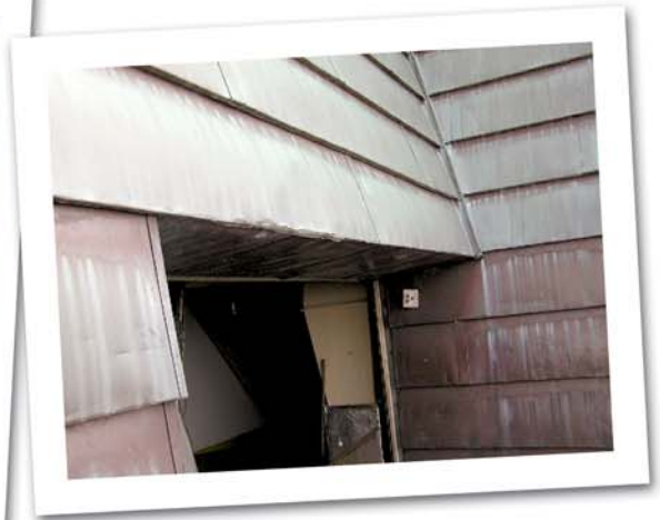
Photo 14: Roll-up door soffit damage.
