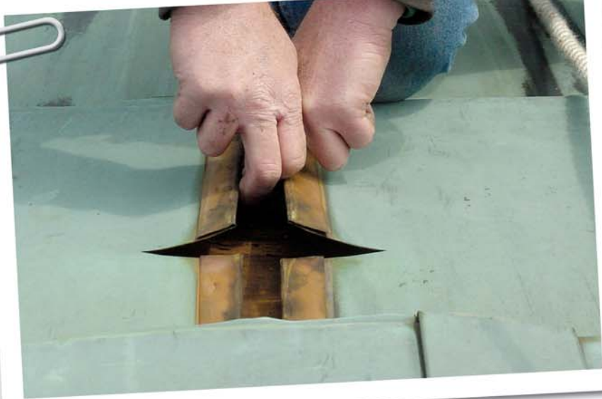
Photo 3: Cracks in copper at drive cleats.
