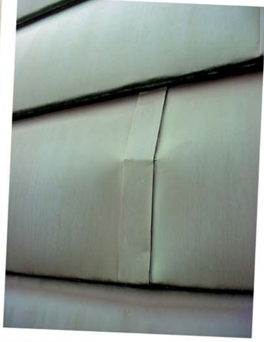
Photo 6: Bowed copper due to accumulation of underlayments (felt and rosin).
