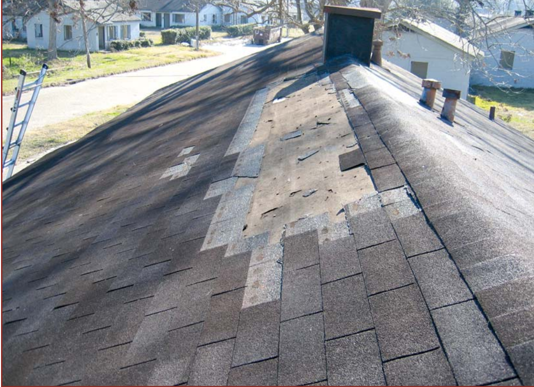
Left: Photo 8 – The most extensive wind loss of shingles occurred near the roof perimeter and with the “old” shingles, such as on Building 13.
