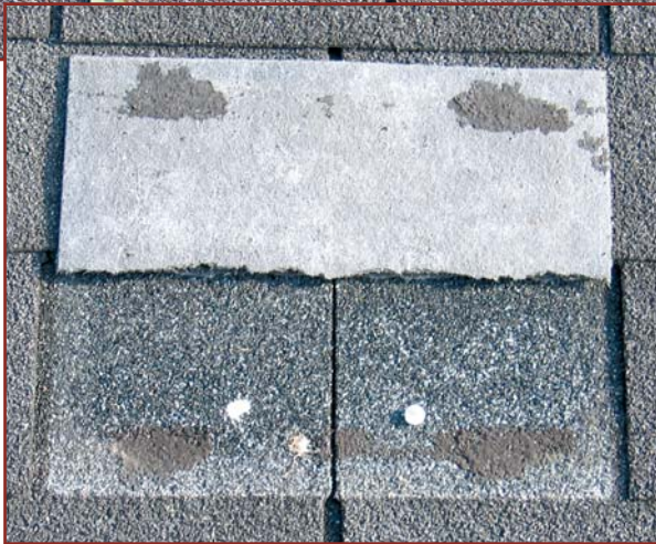
Above: Photo 6 – Nails were underdriven and located too high with the “moderately old” shingle roof installation on Building 2.
