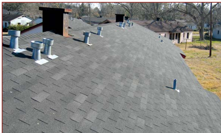
Photo 3 – The center wing of Building 12 had a “recent” shingle roof typical of four buildings within the complex.
