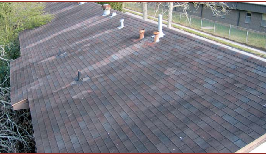
Photo 2 (left) – The long wing of Building 1 had an “old” shingle roof, typical of nine buildings in the complex.
