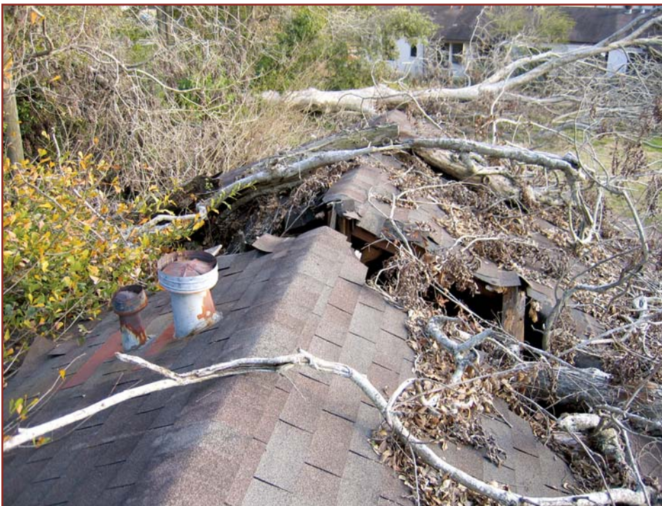
Photo 12 – Although the “old” shingles on Building 3 suffered very little direct wind damage, structural damage from this fallen tree would necessitate replacement of the shingles.
