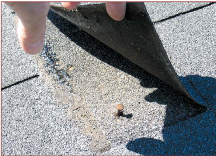
Photo 7 – Nails were underdriven and located too high with the “recent” shingle roof installation on Building 15.
