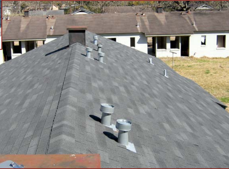
Below: Photo 4 – The long wing of Building 16 had a “moderately old” shingle roof, typical of five buildings in the complex.
