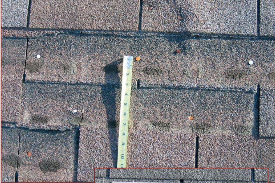
Above: Photo 5 – Nails were underdriven and located too high with the “old” shingle roof installation on Building 10.
