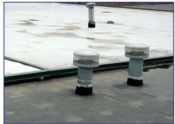
Figure 3 – Photo of roof on December 15, 2003. The PVC membrane is on the top, in white; the EPDM membrane is in the foreground.
