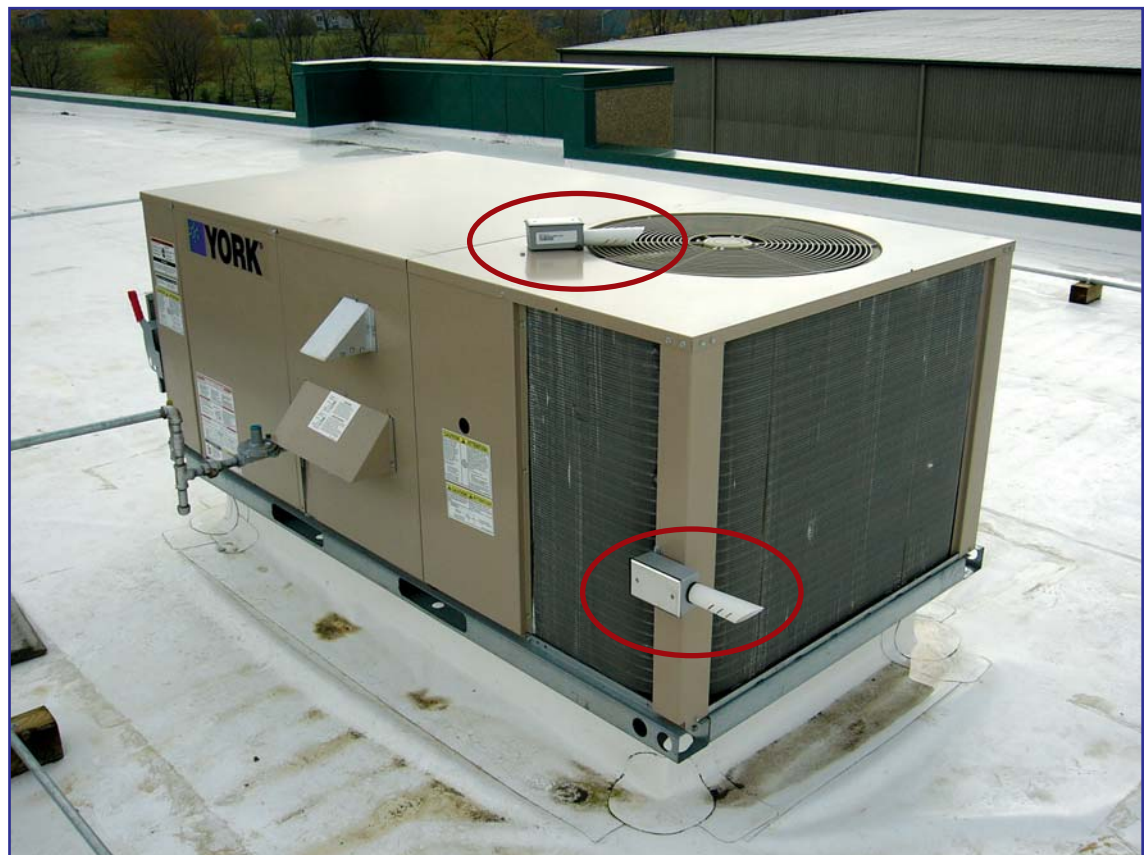
Figure 9 – York HVAC unit with sensors (circled).
