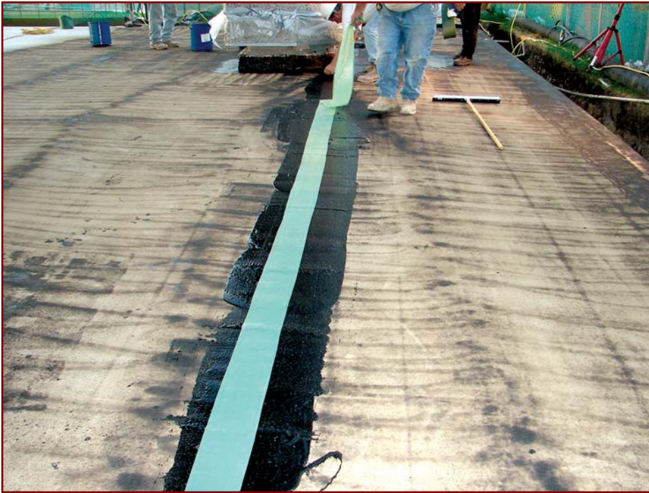
Photo 8: Each manufacturer's requirement for substrate crack treatment varies. Designers should take the most conservative approach in addressing substrate cracks to avoid future problems.
