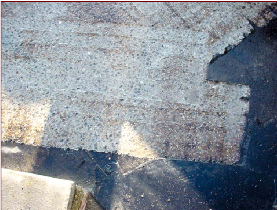
Photo 6: Scarifying is a good method for removal of an existing adhered waterproofing membrane. However, care should be taken to avoid over-roughening of the substrate.
