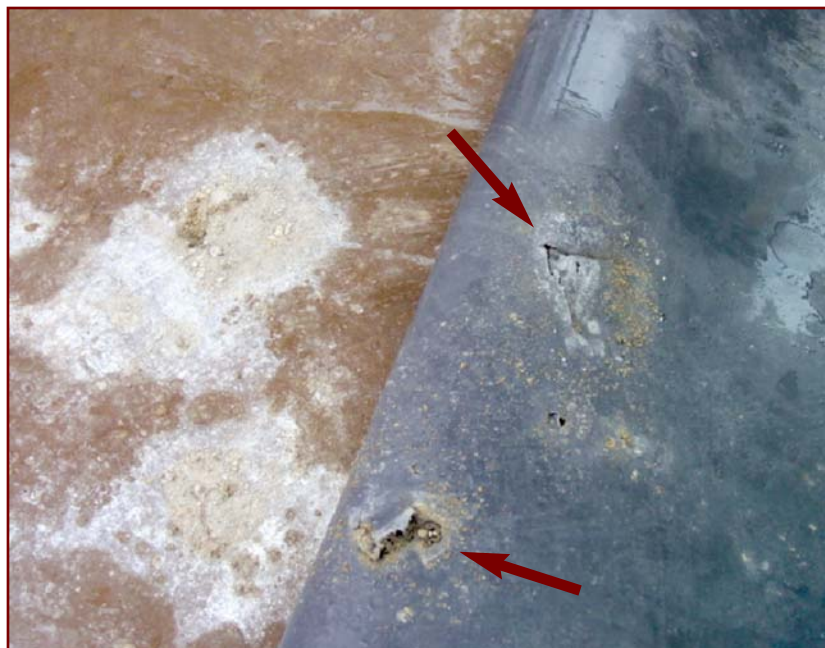
Photo 5: Inadequate surface preparation can lead to problems. Small pieces of gravel left on the surface can lead to punctures in the membrane.
