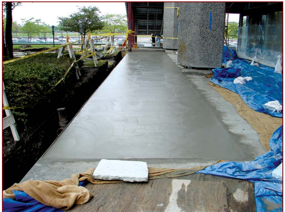
Photo 2: A cementitious tapered topping can be installed in some cases to improve subsurface drainage. Note the previously placed areas to the right are being moist cured with burlap and plastic sheets.
