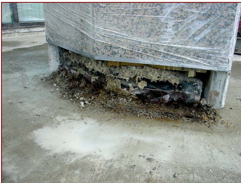
Photo 3: In many cases, original waterproofing system base flashings are installed prior to many exterior components, such as column cladding. In such cases, column claddings and curtain wall bases will have to be modified so that new base flashing can be installed.
