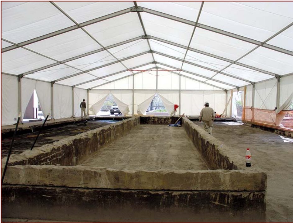
Photo 4: In some cases, the work areas will have to be completely enclosed temporarily to provide weather protection during plaza rehabilitation.
