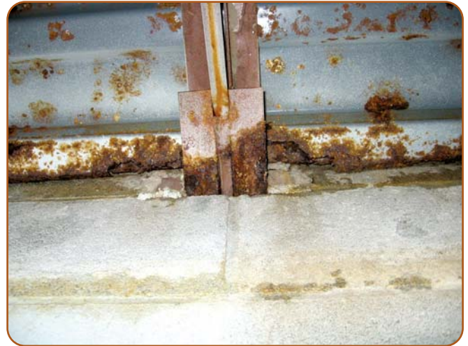
Deteriorated metal decking.
