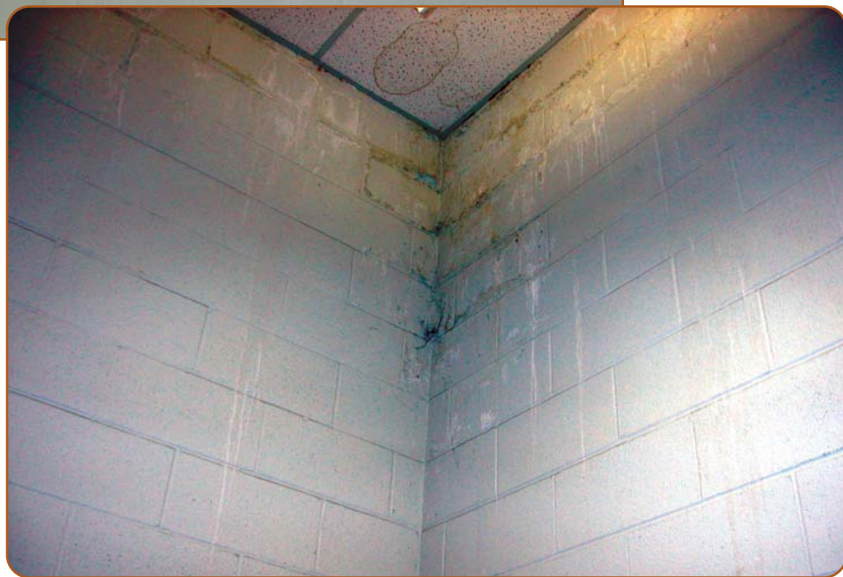
Below: Interior damage.
