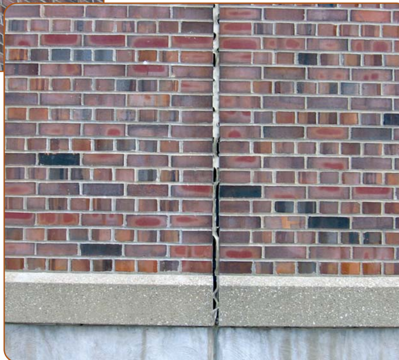
Separated expansion joint.
