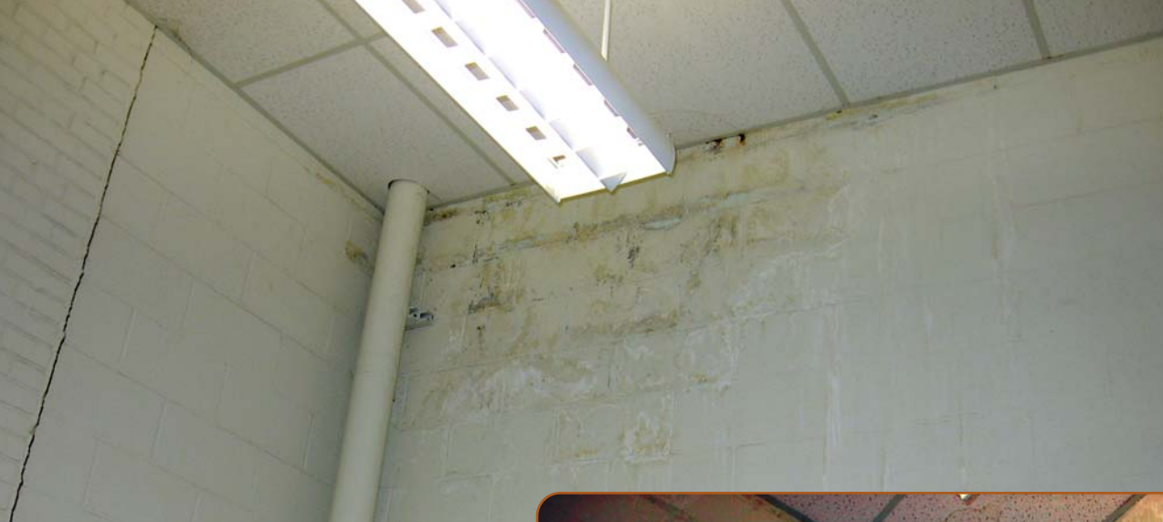
Left: Interior wall and ceiling damage.
