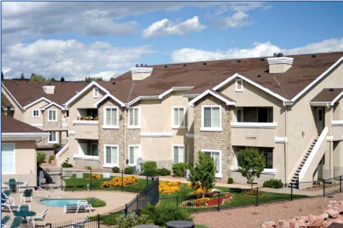
Photo 1. Overview of a building on the property, showing the loss of shingles.
