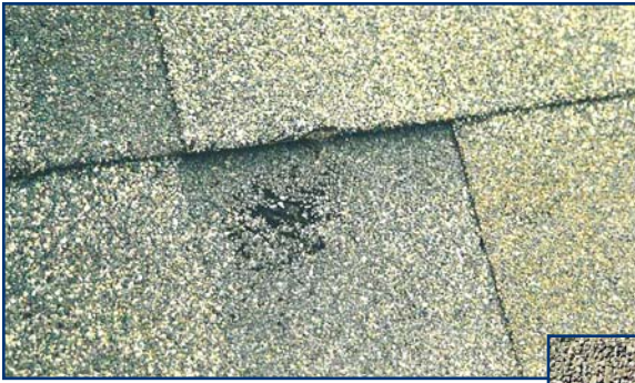
Figure 4 – “Bruising” of the protective granules but no loss of the coating asphalt. Surface temperature at the time of hail has considerable influence on damage susceptibility.
