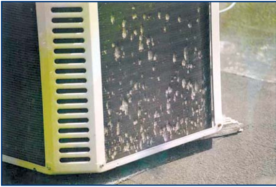
Figure 14 – Deformed cooling fins on HVAC units are the sure signature of hail exposure.
