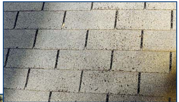
Figure 2 – “Rash blistering” is particularly likely when substandard attic ventilation is afforded. The tiny blisters can rupture under even very light contact, leaving the appearance of small pockmarks.
