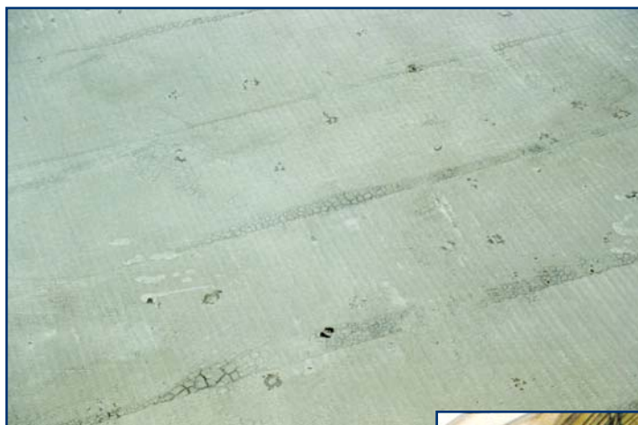
Figure 11 – Roof coating can be compromised by hail exposure, even when the felt plies remain intact.
