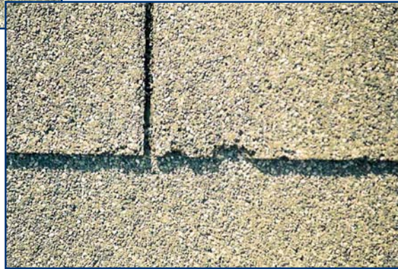
Figure 5 – Chipping of shingles edges (only) with no evidence whatsoever of ordinary pockmarking.
