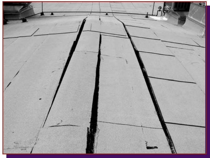
Figure 1. Cap sheet installed on steeper slope with the wrong type of asphalt.
