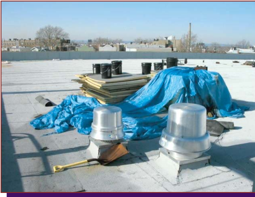
Figure 3. Improperly stored materials should not be used in the construction of a built-up roof.
