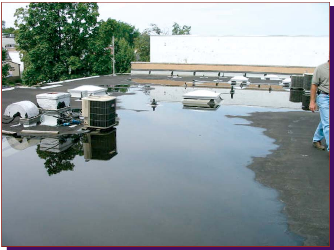
Figure 2. Ponding water reduces the life expectancy of a roofing system.
