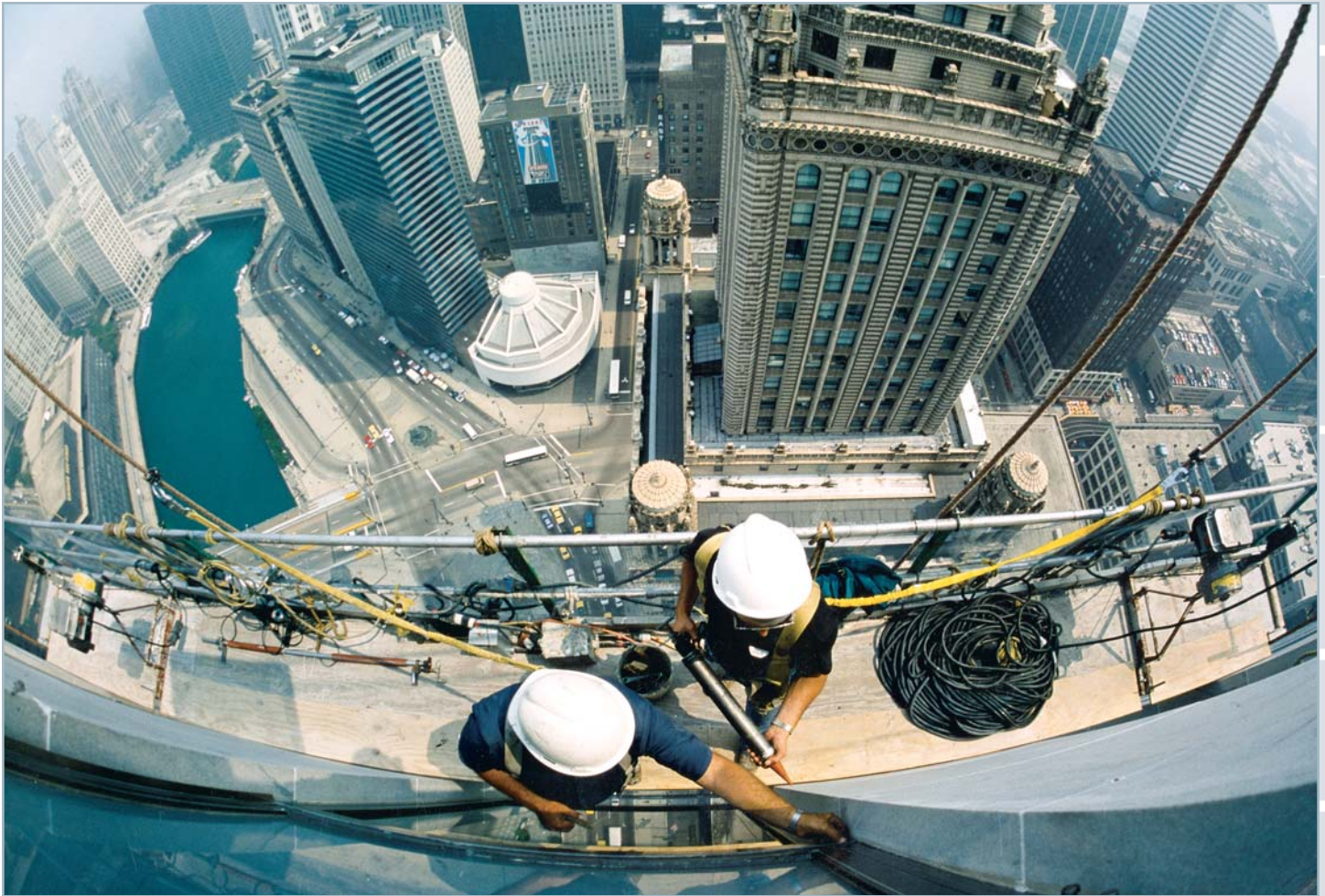
Flying high over Wacker Drive in downtown Chicago, inspectors with Western Waterproofing Co., Inc. work on a building's façade per Chicago's façade inspection ordinance.
