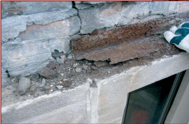
Below: Figure 9 – Heavy corrosion of steel window head lintel. Note the minimal bearing tolerances at the end of the steel lintel and cut limestone “surround” of the window opening.
