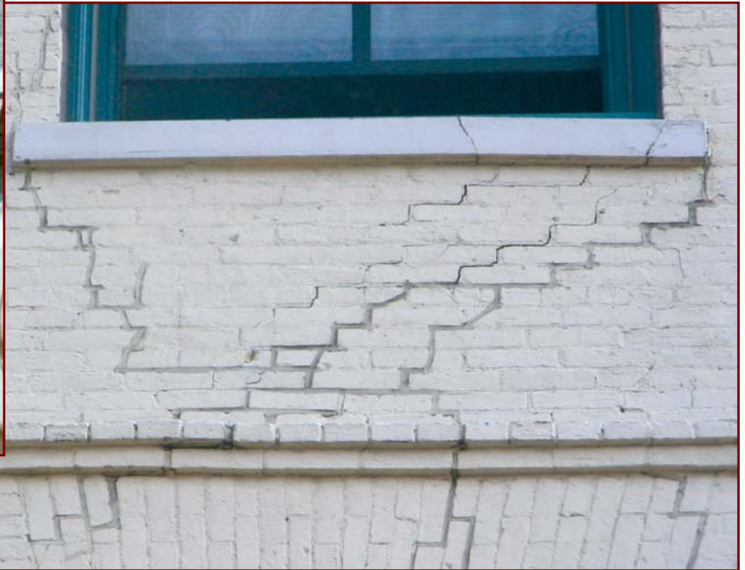
Figure 17 – Stair cracking common to window openings in solid wall construction.
