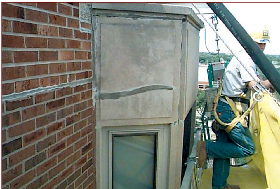
Figure 3 – Area of localized distress in cut limestone cladding.
