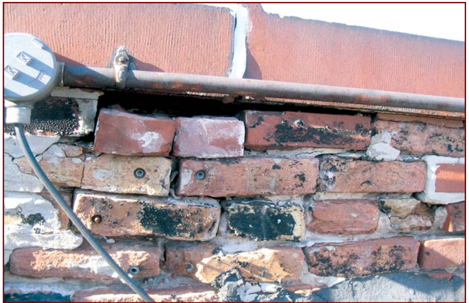
Figure 6 – Typical conditions observed on the inboard face of multiple-wythe parapet wall.
