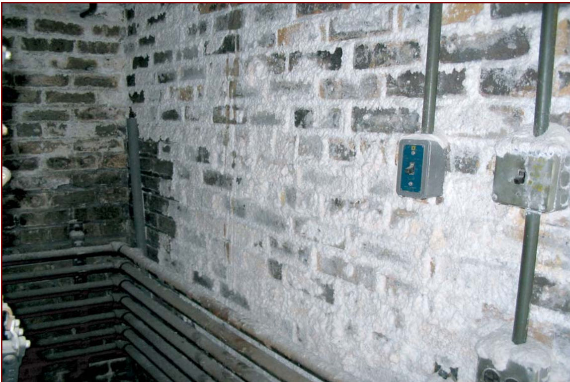
Figure 12 – Heavy concentration of efflorescence on the interior of outside walls is a clear indicator of moisture infiltration.
