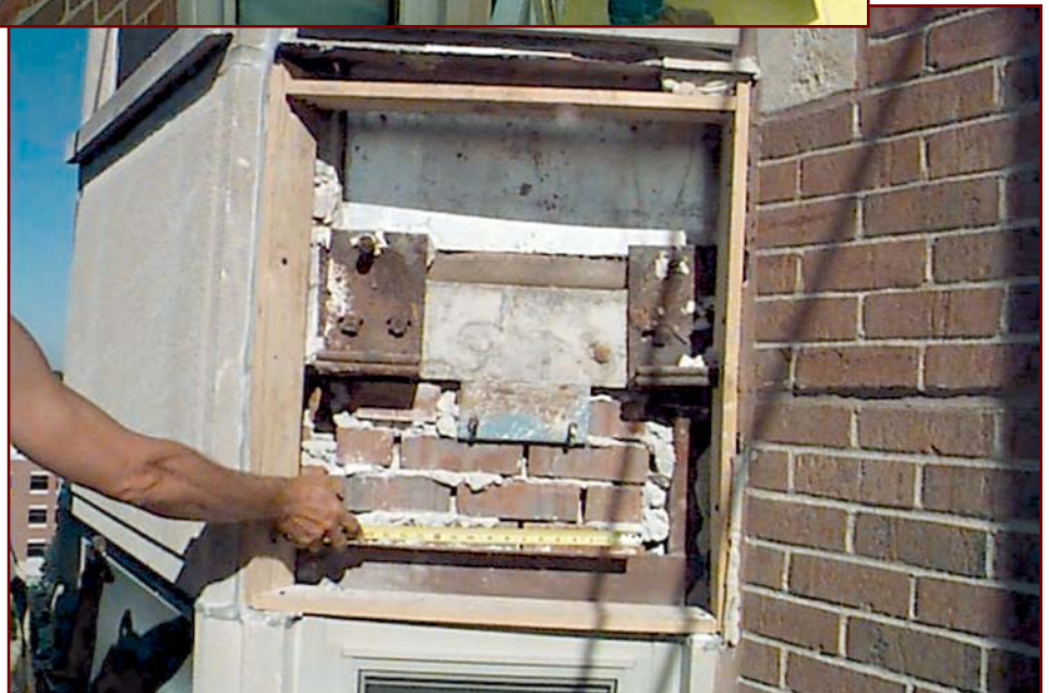
Figure 4 – Inspection opening to establish as-built condition(s) contributory to the cause of the distressed cladding feature.
