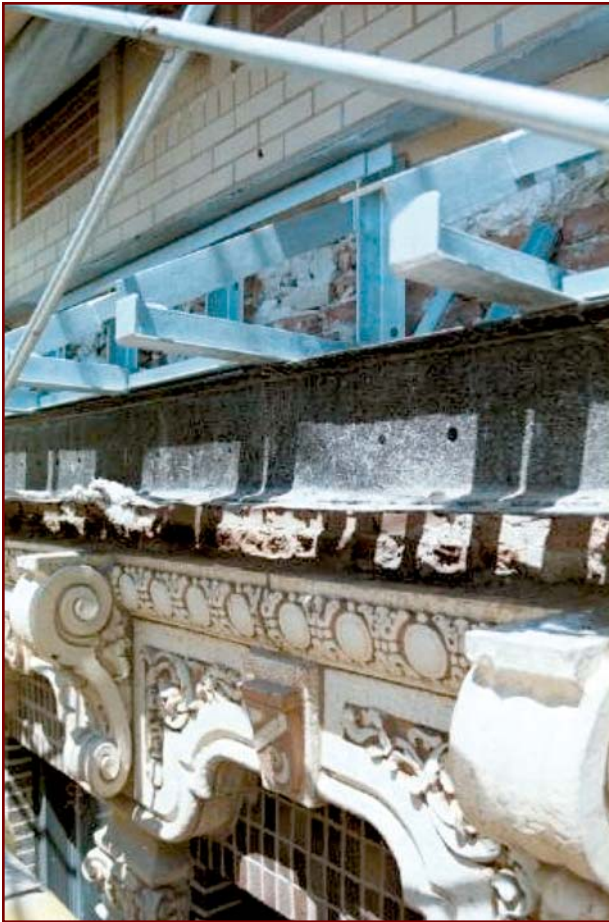
Figure 16 – Mock-up in area of removed terra cotta cornice with new steel framing intended as anchor points for replacement GFRC.
