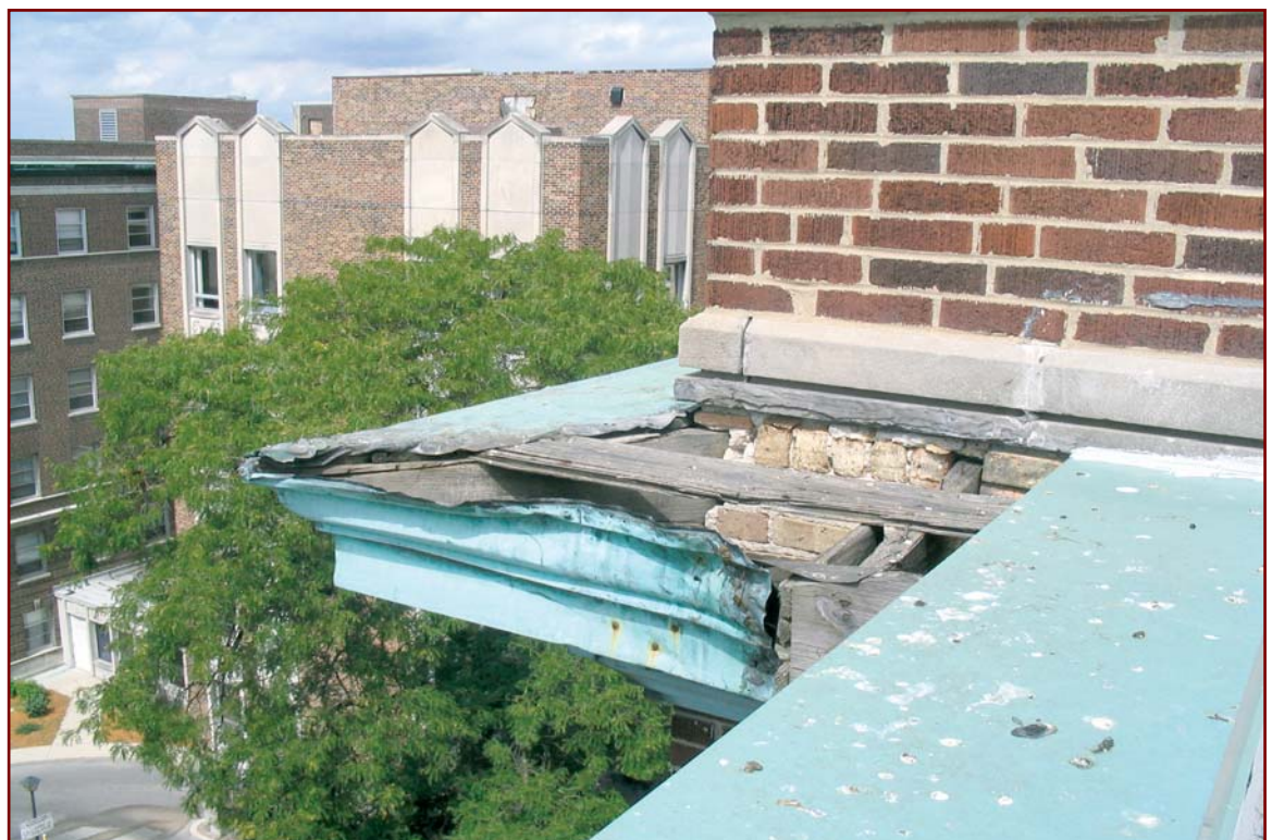
Figure 13 – Damage to wood-framed, copper-clad cornice feature.
