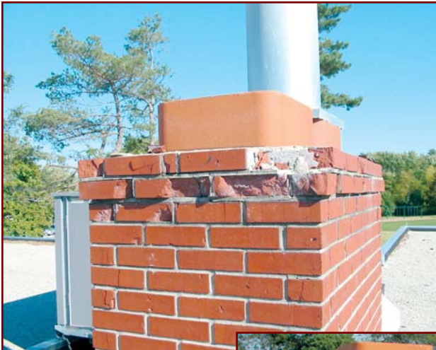
Left: Figure 11A – Typical chimney damage due to water infiltration and subsequent freeze/thaw damage (2002).
