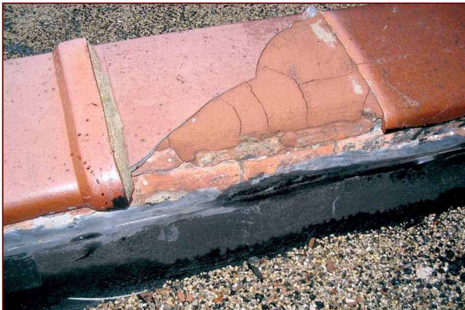
Figure 7 – Typical, overall poor condition of above-roofline parapet wall and coping.
