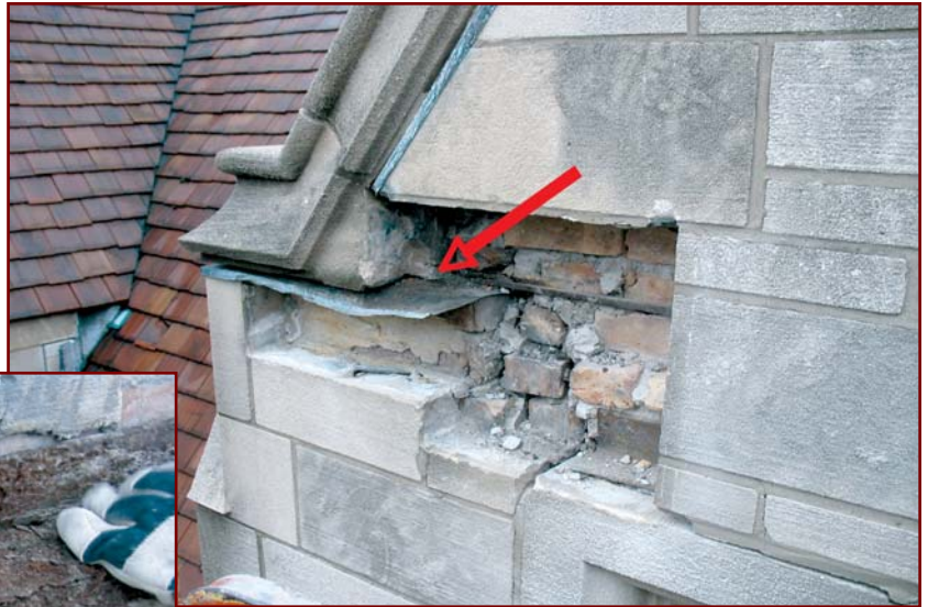
Figure 8 – A lack in continuity of the 1930s-era through-wall flashing below the stone coping resulting in out-of-plane conditions.
