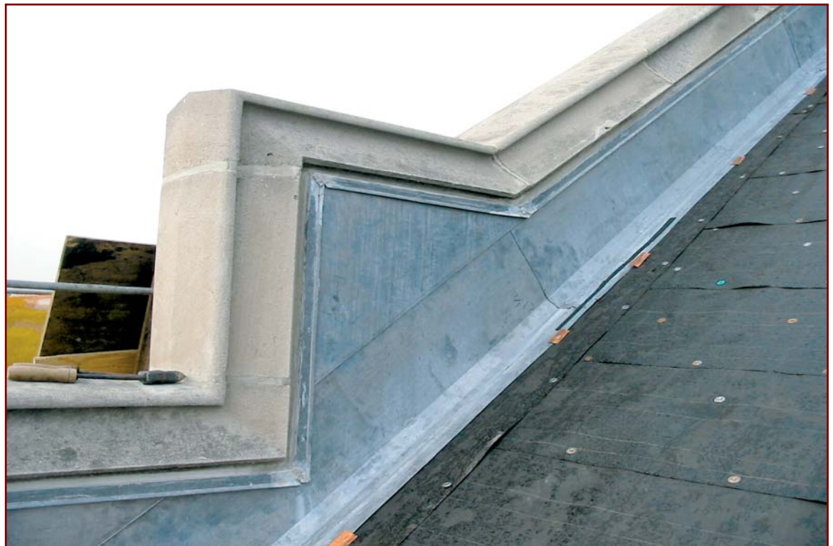
Figure 10 – Above-roofline masonry offered protection by sheet metal cladding interfaced with a new, continuous through-wall flashing below the limestone cladding.
