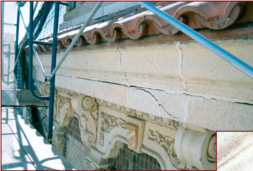
Left: Figure 14 – Terra cotta cornice classified as in an unsafe condition.
