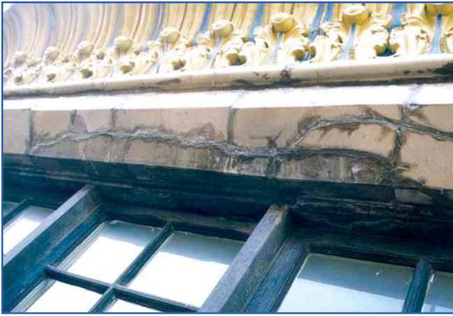
Figure 1 – Cracked masonry over a window opening is a typical condition façade inspectors should identify and classify. Knowledge of the exterior wall type is required in order to classify the condition.
