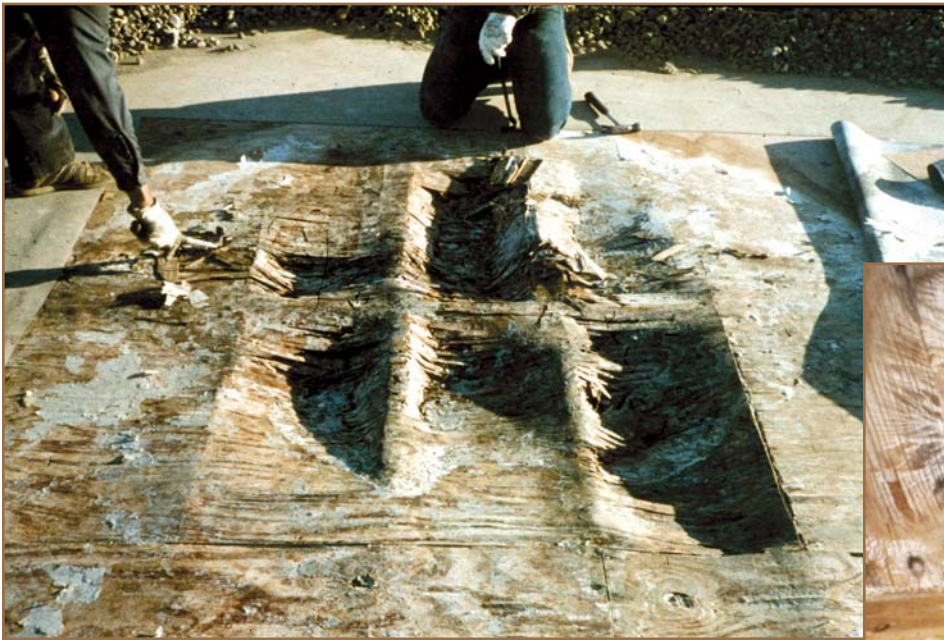
Photos 7 (left) and 8 (below) – Severe plywood deck deterioration with fungi growth caused by condensation over a laundry room in multi-family apartment building.
