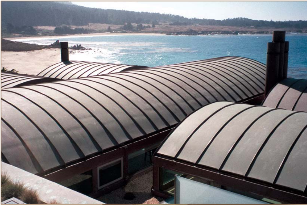
Photos 5 (left) and 6 (below) – Saturated plywood sheathing below self-adhering membrane underlayment in a non-vented barrel roof with a standing seam copper covering.
