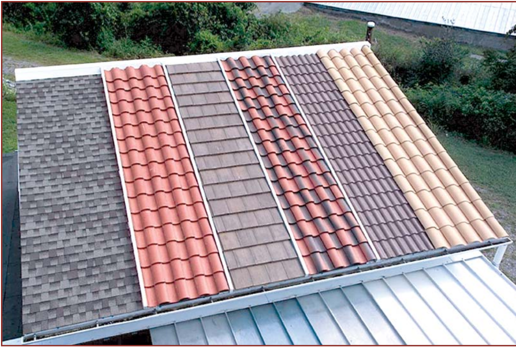
Figure 2 – An assembly of steep-slope attics was placed on top of the ESRA. Clay and concrete tiles were installed by the Tile Roofing Institute.
