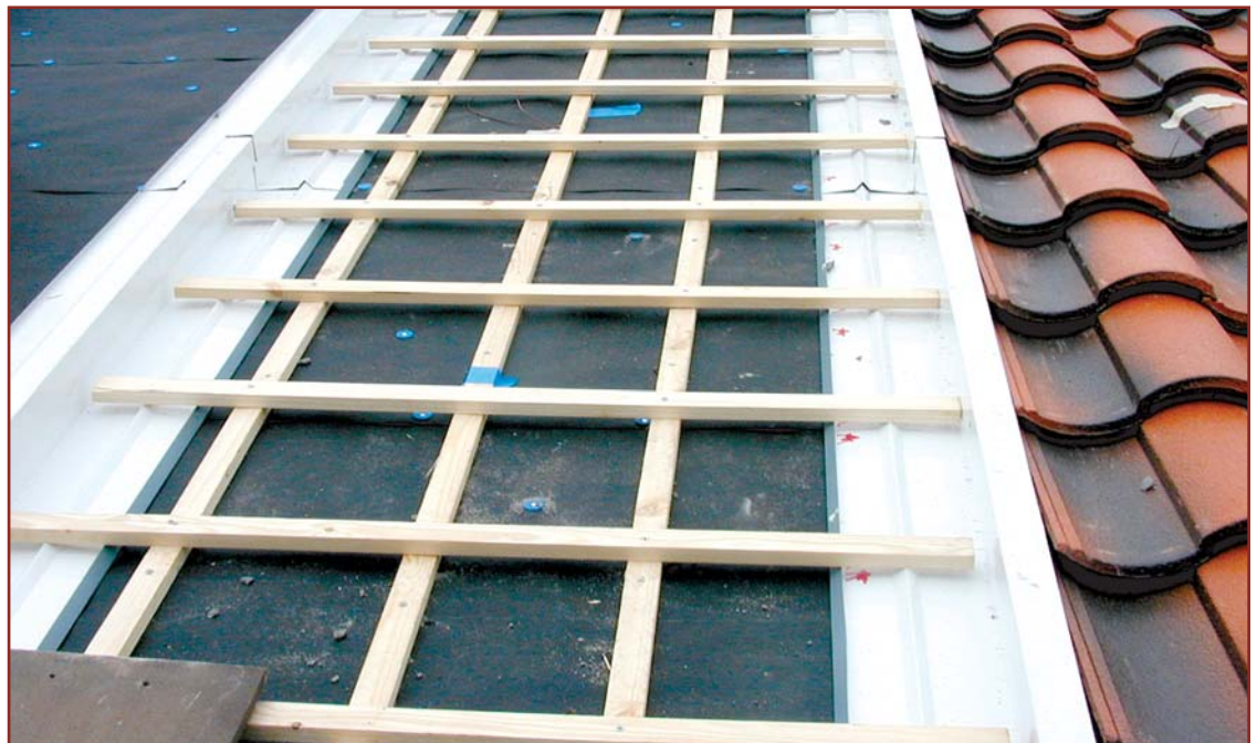
Figure 3 – Construction of the roof deck showing battens and counter-battens for attaching the slate tile. The parapets are used to limit airflow on the underside of the tile to within a given test roof.
