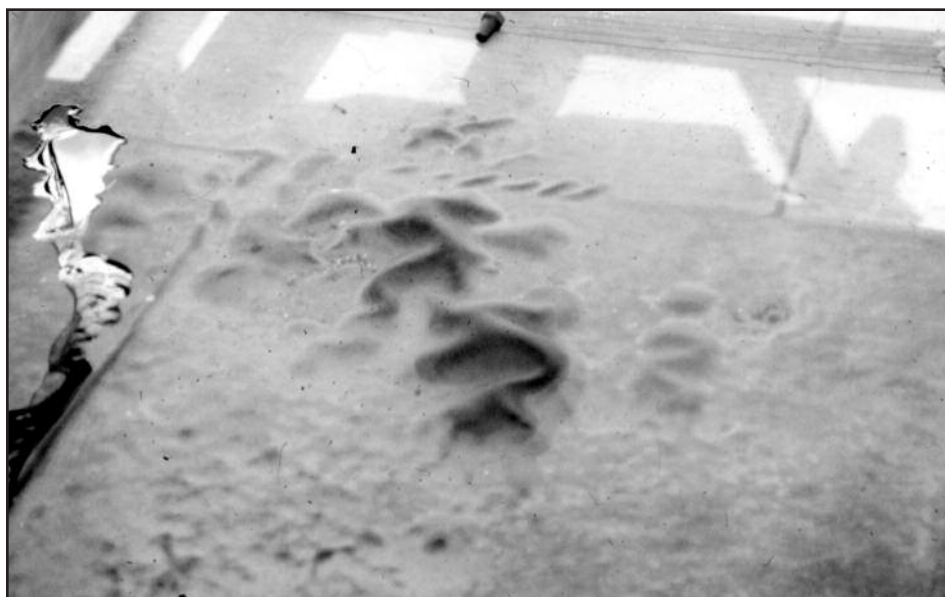
Photo 2 - Swelling of liquid-applied membrane.
