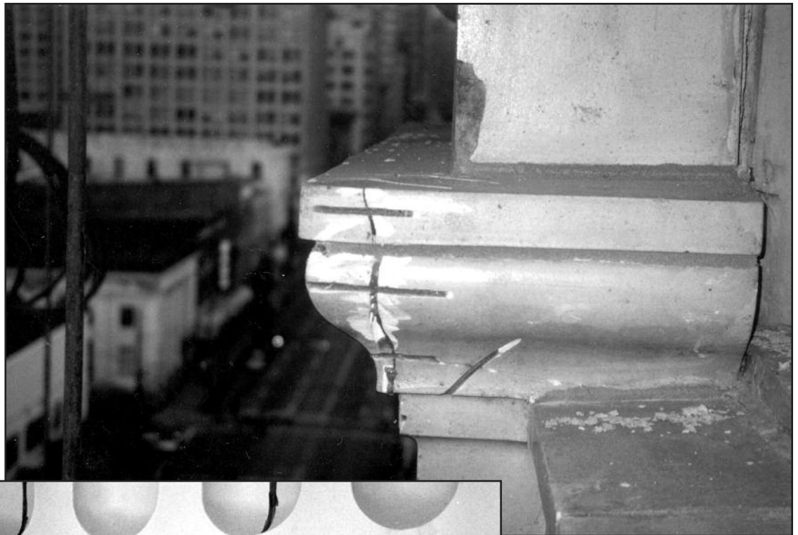
Figure 6 – Pinned terra cotta unit.
