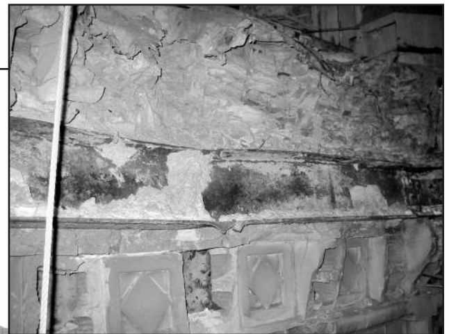
Figure 7 – North facade – impact damage crushes terra cotta, bends, and nearly shears through a steel spandrel beam.
