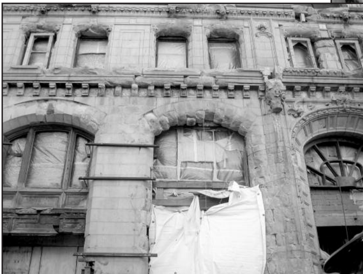
Figures 17A and 17B – North granite base – fire and impact damage rendered much of the north base unrestoreable.
