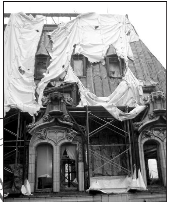
Figures 13A and 13B – Mansard roof – copper sheets melted and wood nailers burned from fire.
