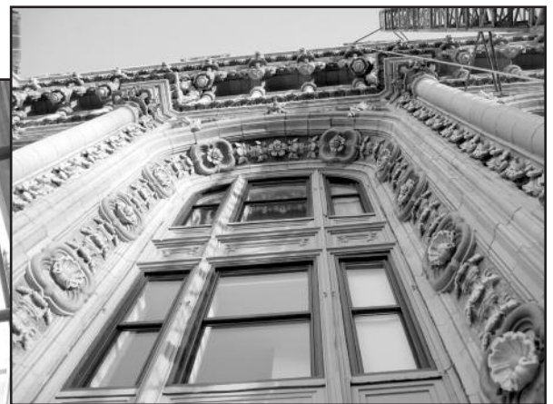
Figure 11 – North elevation – completed restoration of devastated area at top of north elevation.
