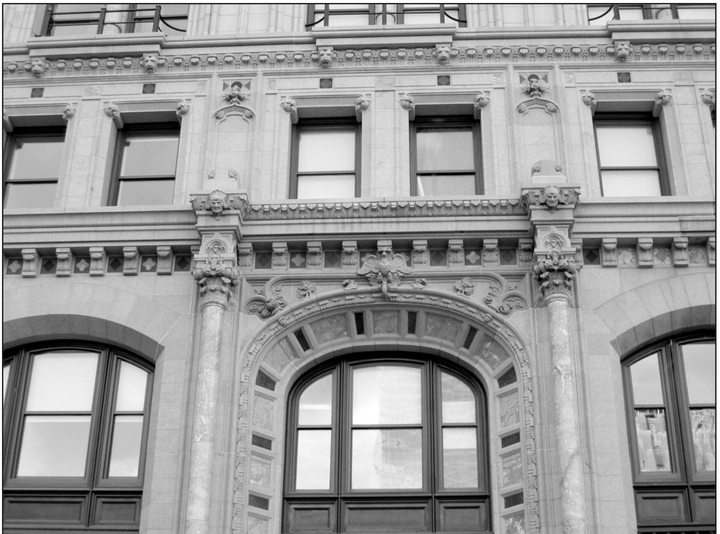
Figure 24 – Completed project – northwest corner, December 2005. Completed north entrance arch where approximately 50% of the original granite was reinstalled after being refitted onto the new panels.
