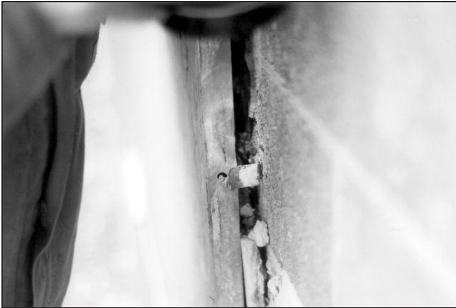
Figure 9 – Outer portion of steel clip engaging stainless steel pin is completely corroded away.
