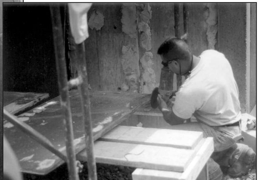
Figure 26 - Removal of existing sealant from edge of slate panel prior to reinstallation.
