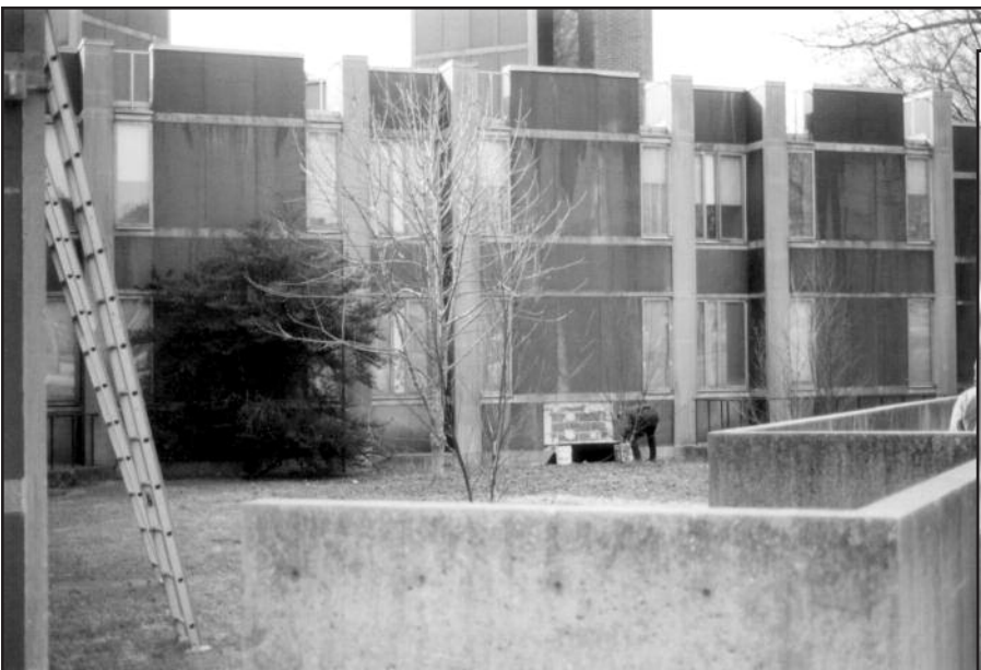
Figure 17 – Embrasures before rehabilitation.
