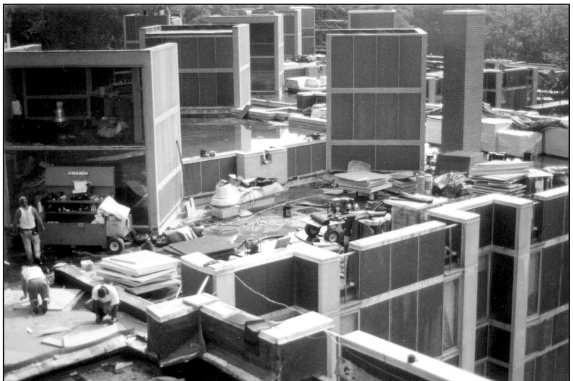
Figure 23 – Puddling on roof during construction.
