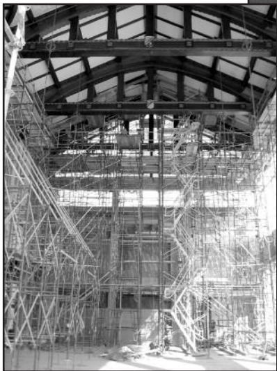
Figure 10 – Main hall with scaffolding to support trusses while end-bearing timber is replaced where rotted from contact with masonry.
