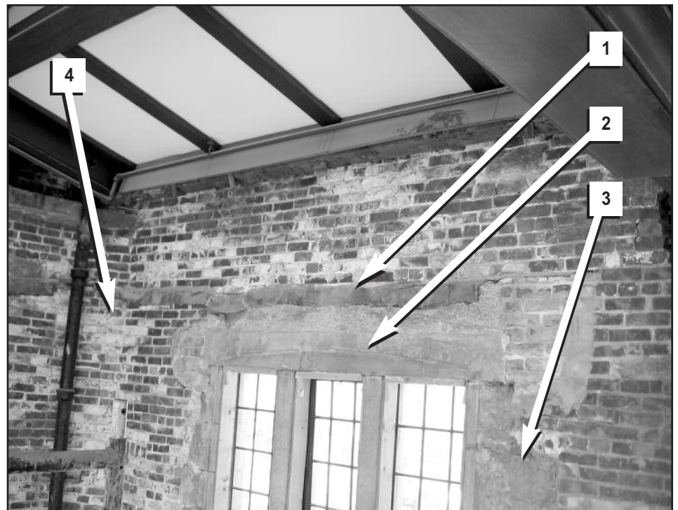
Figure 2 - Interior of masonry wall showing damp-proof (1) course above window lintel (2), bond stone (3), and efflorescence on masonry (4).
