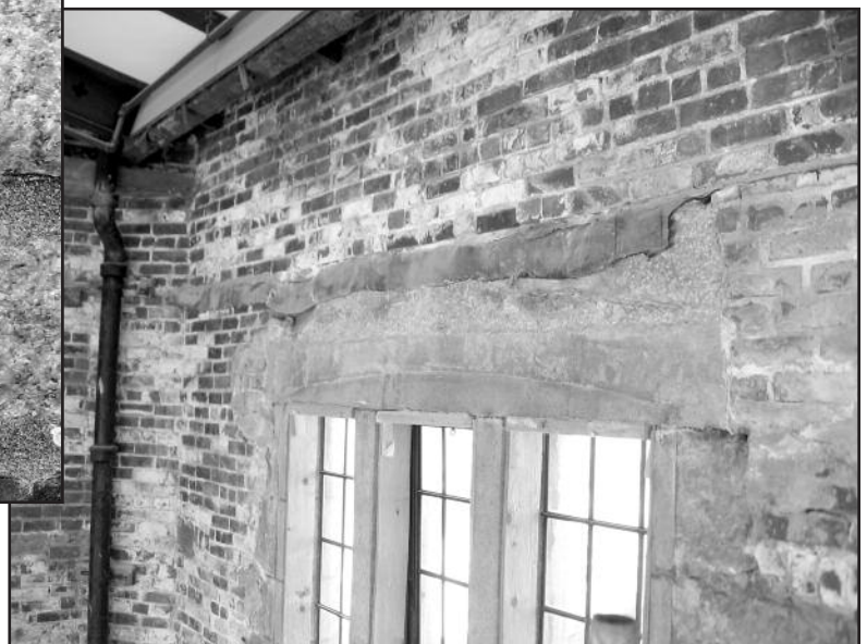
Figure 9 - Efflorescence on interior face of wall showing location of long-term evaporation of water from the brick.
