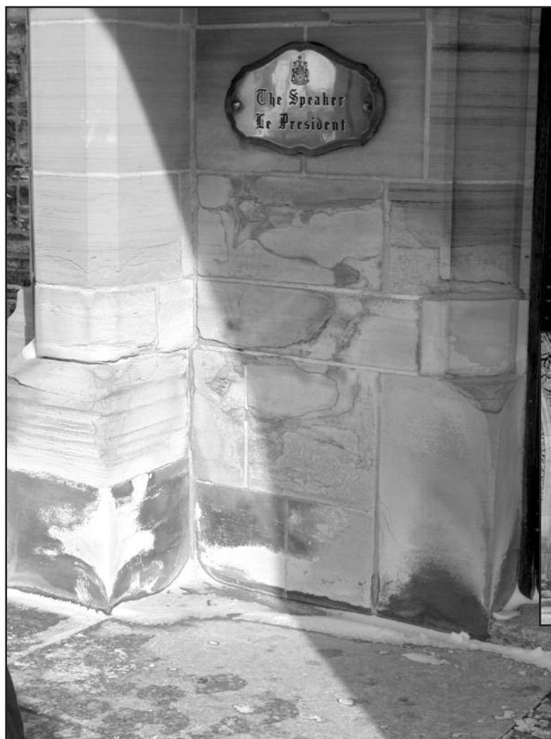
Figure 3 – Salt damage to stone and mortar is apparent beside an entryway where salt is used to remove ice in the winter.
