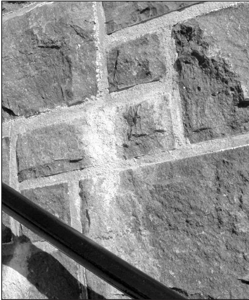
Figure 5 - Lime leached out of the mortar joints onto the masonry surface leaves an unsightly stain. Had the lime had chance to carbonate before being exposed to the weather, this might not have occurred.
