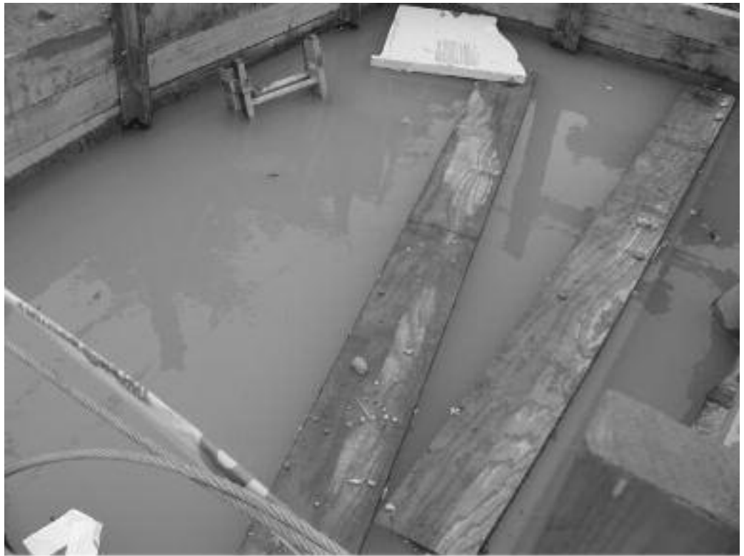
Dewatering responsibilities must be delineated prior to start of work. Note the ladder in the water.
