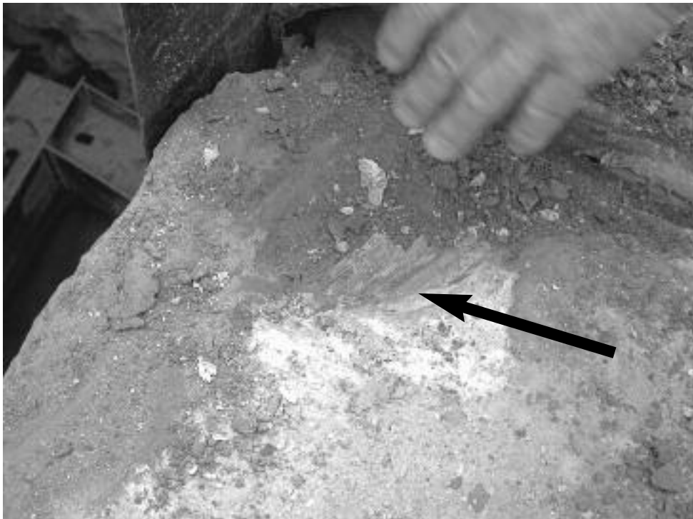
Water stop that migrated up into the concrete slab during the initial pour. Concrete at corner of expansion joint subsequently spalled, causing joint leakage.
