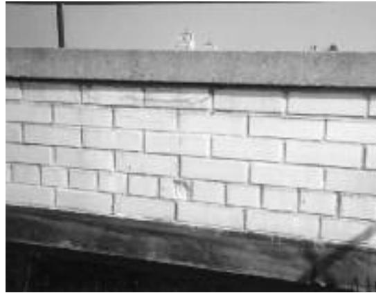
Figure 2 – Freeze-thaw distress at parapet.
