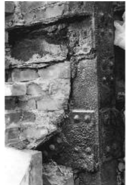
Figure 3 – Rust scale on structural steel.
