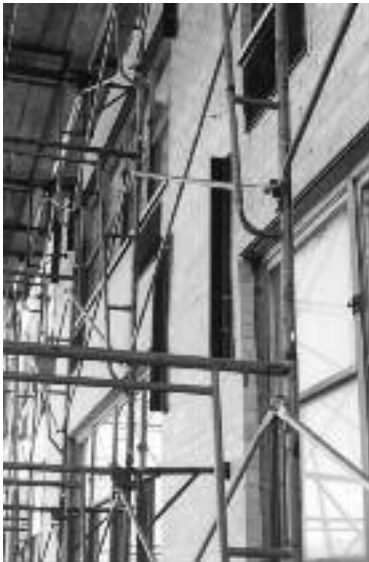
Figure 9 – Temporary bracing angles used to prevent bulged masonry between windows from falling.
