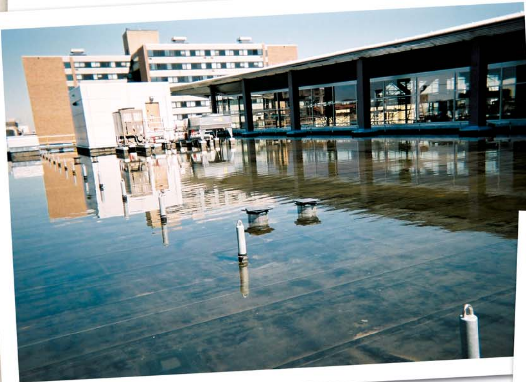
Above left: The green roof basin is flooded to test the waterproof seal.
