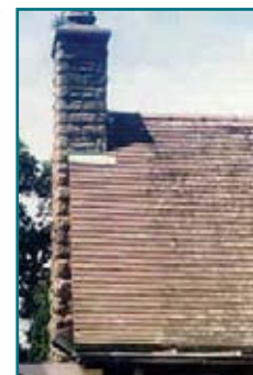
Figure 2: This roof, on a golf course clubhouse in South Africa, shows that Gloeocapsa Magma is as much at home in Africa as North America. Also note the effect of the copper flashing around the chimney. (Courtesy, Michael Rosenthal, Durban, South Africa.)
