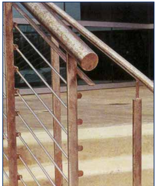
Figure 2 – Stainless steel railing corrosion. (Photo courtesy of TMR Stainless.)
