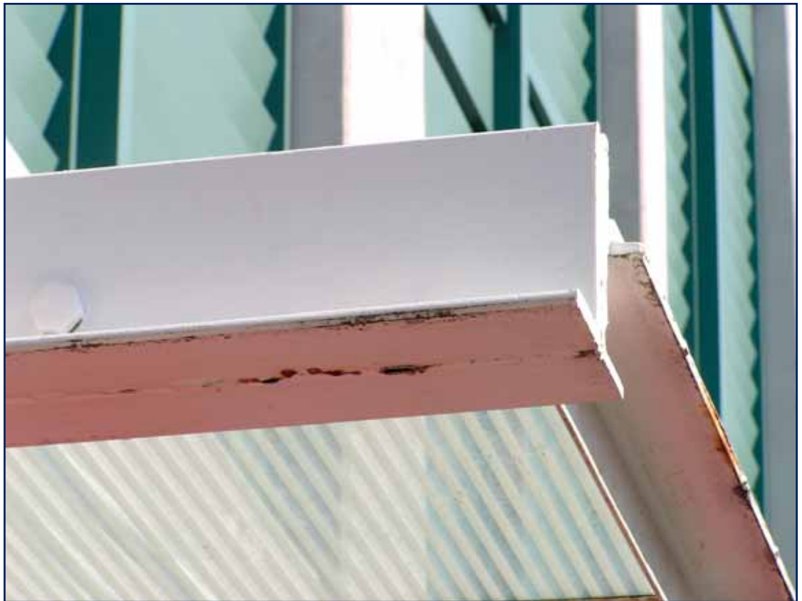
Figure 6 – Shop primer failure.
