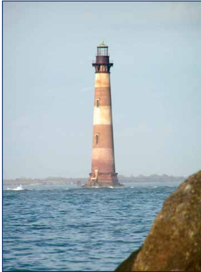
Figure 5 – Lighthouse with discolored paint.
