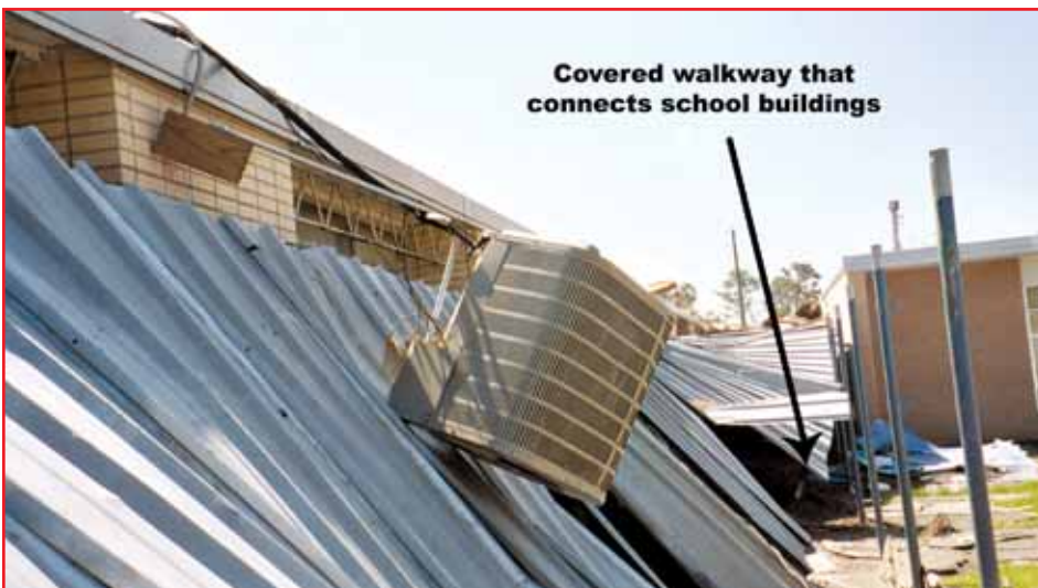
Photo 9 – A roof-mounted air conditioning system landed on a covered walkway.
