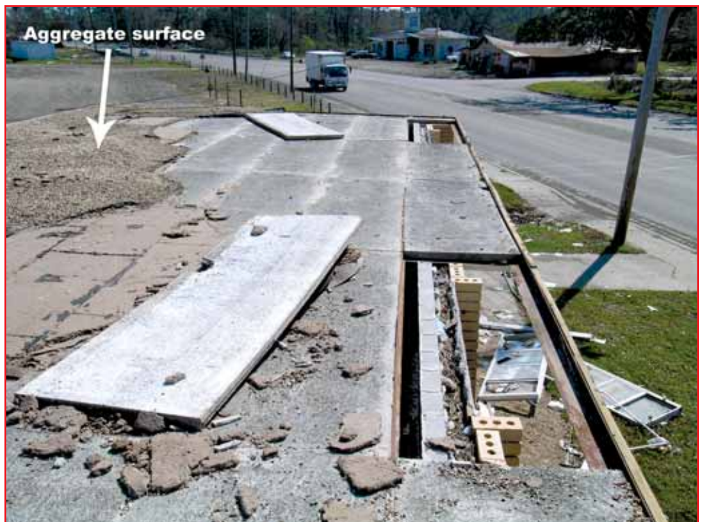
Photo 7 – This four-ply, aggregate-surfaced, BUR system suffered 95% membrane damage.
