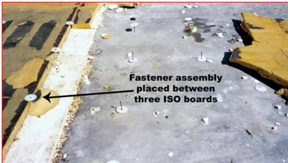
Photo 5 - Fasteners were driven between ISO sheets, shared by adjacent boards.
