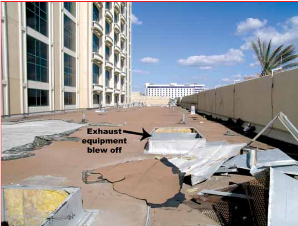
Photo 6 – Developing and following a prescribed method to secure HVAC systems to curbs could reduce membrane damage from equipment dragged or thrown by the wind.
