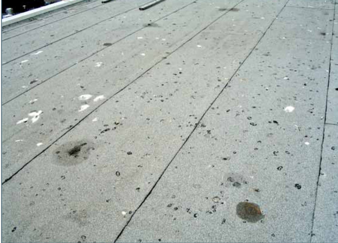
Photo 6 – This photo was taken after the roof had been well washed by rain. The small, round marks are typical of granule loss damage to modified bitumen membrane caused by gull droppings. The larger, “splotchy” marks exhibit damage to the actual membrane, down to the reinforcing, in some locations. Some of what these birds eat and defecate dissolves or softens asphalt!
