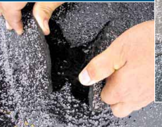
A metal fastener in the gypsum deck where the lightning hit.
