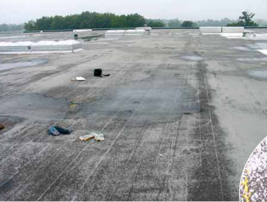
The open area where the lightning struck in several spots.
