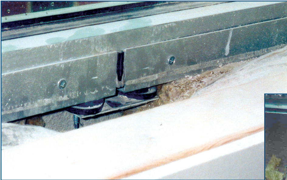
Photo 7 – Up-close view of a splice joint in a sub-sill (viewed from interior, with interior finishes removed). Note the corrugated profile of the splice material.
