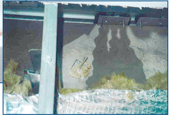
Photo 8 – Heavy leakage is shown through a splice in the sub-sill (shown in Photo 7) due to failed seal with irregularly spliced material (viewed from interior and below, with interior finishes and insulation removed to expose the leakage).
