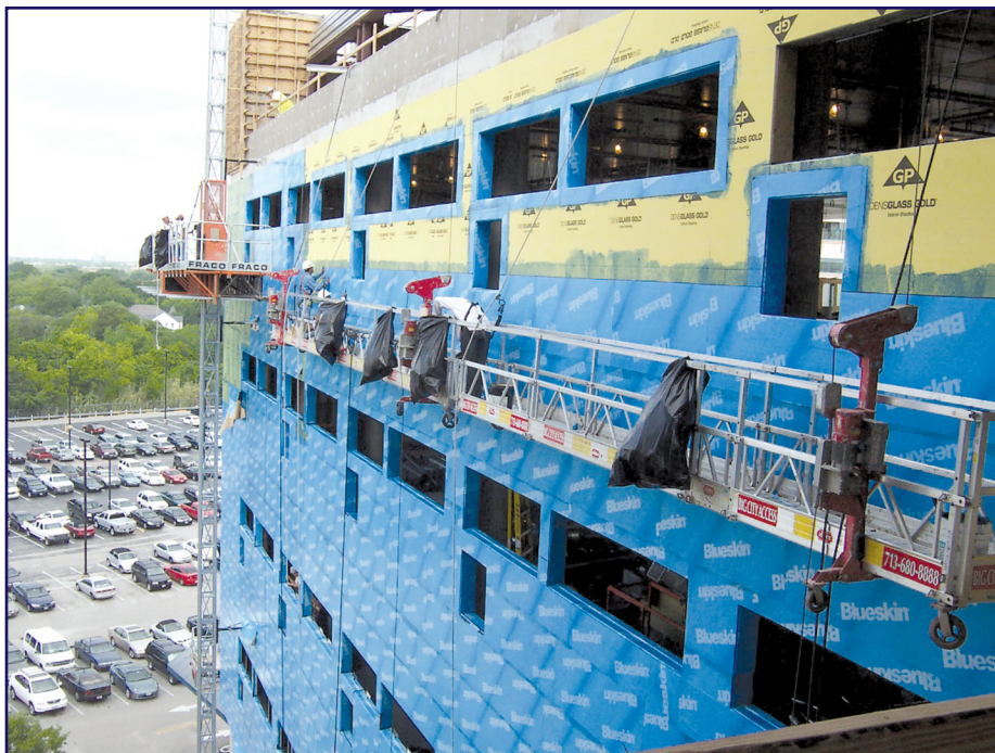
Photo 3 – Project near completion showing a properly prepared wall with subsequent installation of the primary air barrier membrane proceeding up the wall in a logical sequence.
