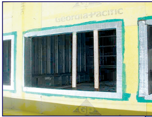
Photo 1 – Air barrier system being installed at the Iowa State University Bio-Sciences Building. The properly detailed window opening uses a UV-stable transition membrane. Note that the wallboard joints have yet to be sealed.
