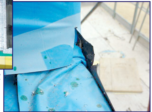
Photo 2 – Air barrier system being installed at Shared Medical Systems, Great Valley, PA. Some would think of this as a good detailing of the opening, but it obviously is not. This usually occurs as a result of starting the project with no assistance from the manufacturer.
