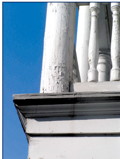
Figure 3-1 – Wood columns painted with an oil-base system and ravaged by years of weathering. The wood in the background is somewhat protected and does not seem to be experiencing the weathering as in the foreground. Photo by Nick Galizia.
