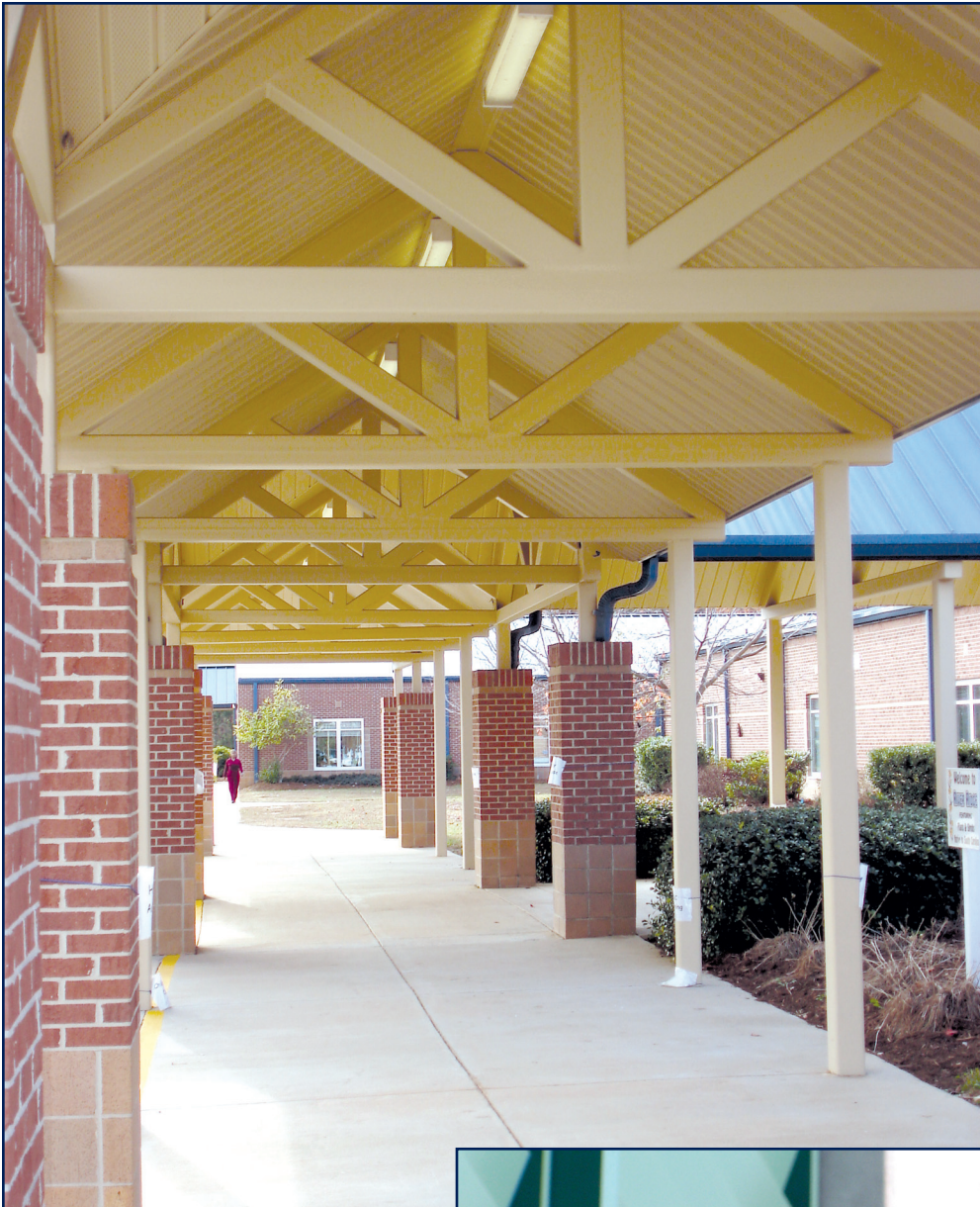
Figure 3-5 – Carbon-steel supports coated with epoxy primer and polyurethane finish after approximately seven years' service. Although the steel is under cover, salt-laden moisture can collect in crevices and on flat areas. This system should maintain its appearance for another seven-plus years.
