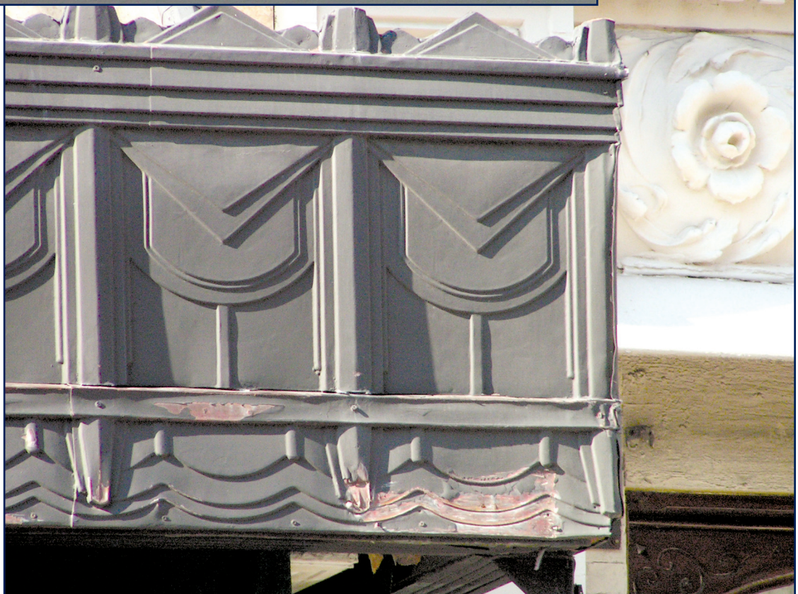
Figure 3-11 – Stamped copper facing that was field painted with an oil-based paint. Paint is faded, curling, and delaminating. Photo by Nick Galizia.
