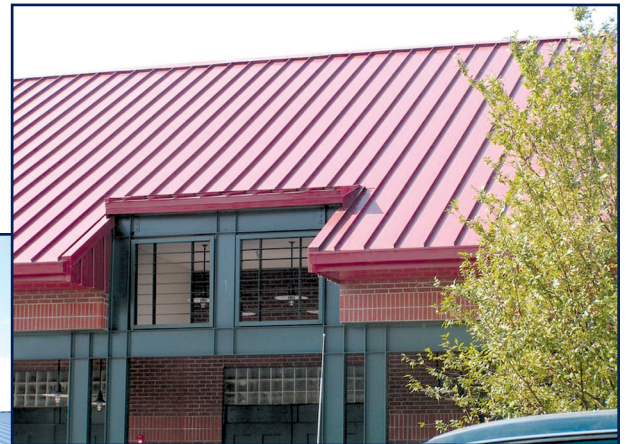
Figure 3-4 – Standing seam roof with fluoropolymer finish over galvanized that is showing excellent performance, color, and gloss retention after prolonged exposure. Photo by Nick Galizia.
