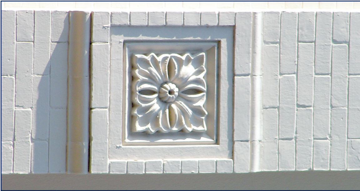
Figure 3-10 – Exterior brick wall painted with alkali-resistant primer and 100 percent, high-performance acrylic. Finish is still sound with little sign of weathering after years. Photo by Nick Galizia.
