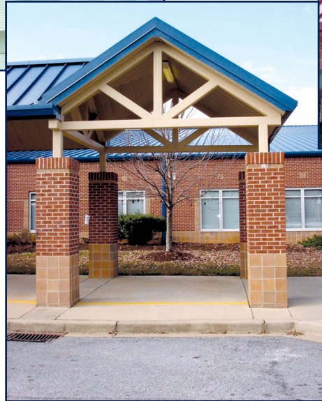
Figure 3-3 – Steel support with epoxy primer and polyurethane finish and steel standing seam roof with fluoropolymer finish. In excellent condition after approximately seven years' service.
