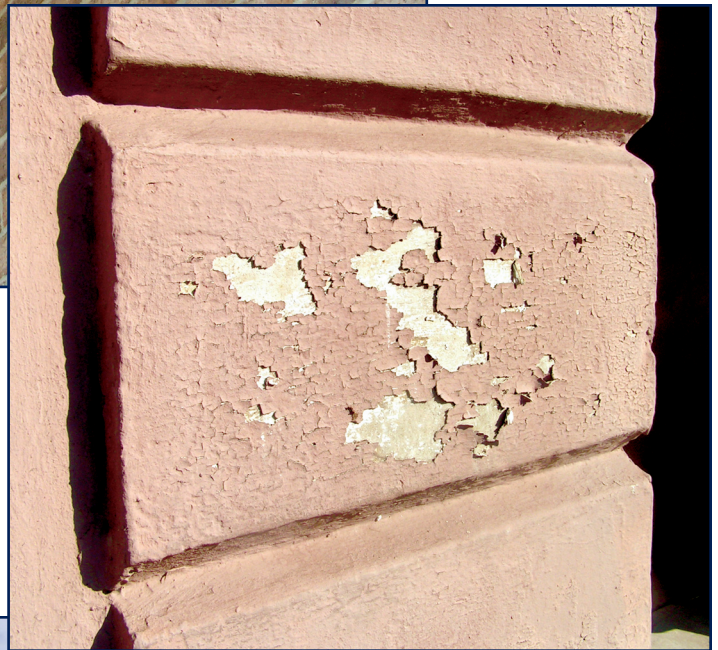
Below: Figure 3-8 – Precast concrete painted with an oil-based paint. Delamination due to moisture within the concrete.
