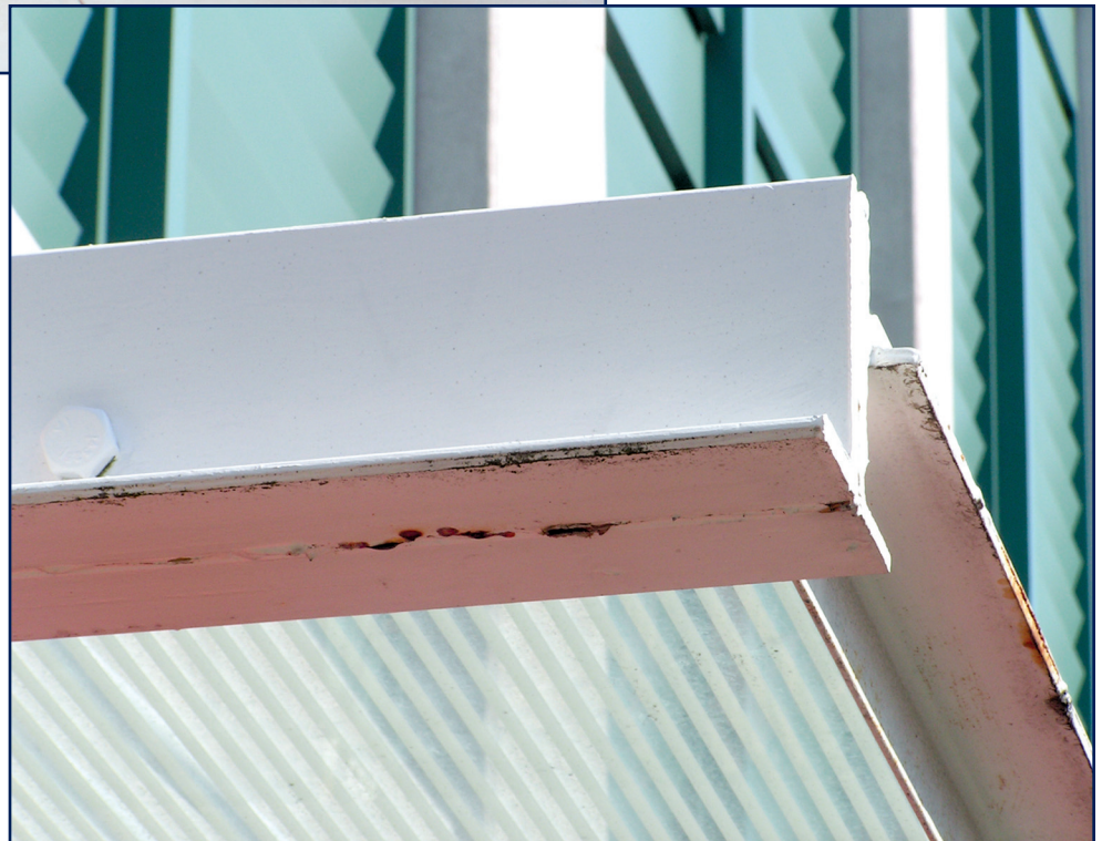
Figure 3-6 – Failure of shop primer before being top coated. The edges of the steel were not stripped to increase primer thickness when the primer was applied. The rust will probably be painted over. Photo by Nick Galizia.
