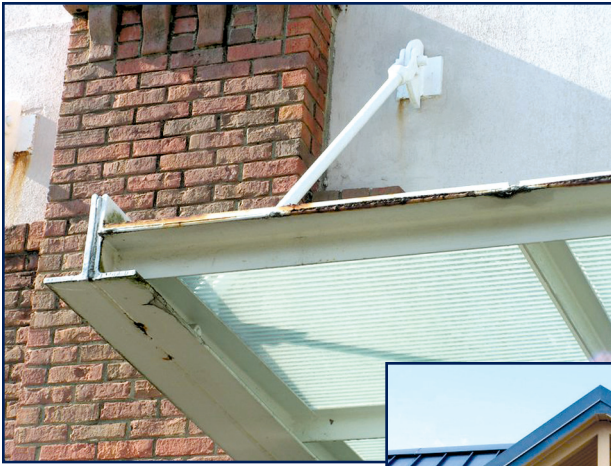
Figure 3-2 – Steel framing that received inadequate surface preparation. The edges were also not stripped in during painting. Insufficient maintenance painting has taken its toll. Photo by Nick Galizia.
