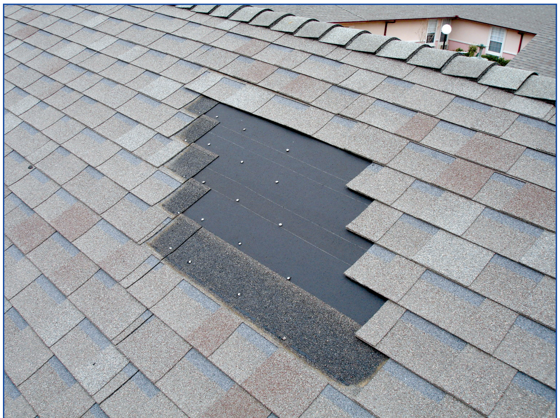
Photo 1 – Shingle failure. Note high placement of nails.
