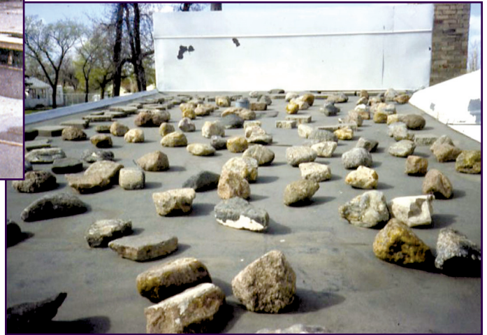
Figure 24: King-sized ballast on this roof!
