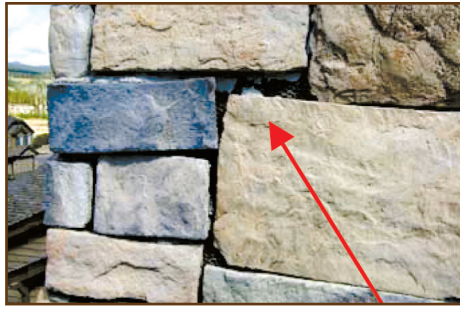
Figure 5: Worst-case scenario. Note missing scratch coat between stones.
