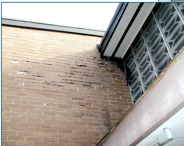
Figure 6: Faulty flashing leads to moisture accumulation and permanent freeze/thaw damage at roof interface.
