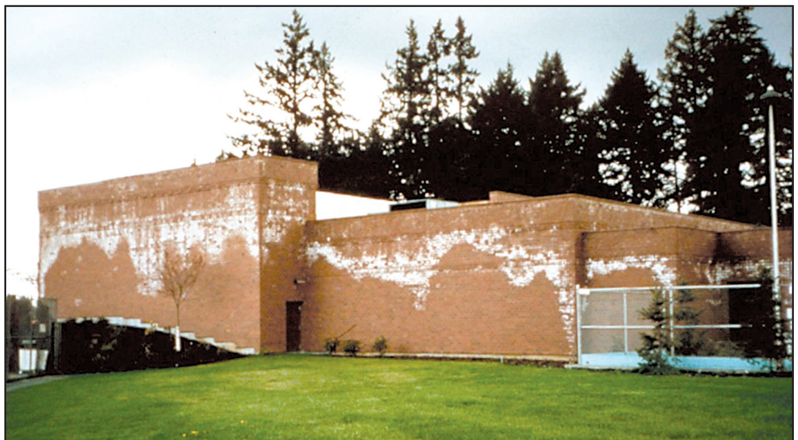
Figure 9: Efflorescence from rainwater penetration can quickly mar a beautiful new masonry façade. (Photo courtesy of Prosoco.)
