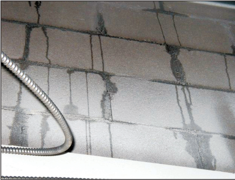
Figure 10: Single-wythe CMU: Interior view of integrally waterproofed CMU block and mortar. The head joints were not properly consolidated and did not prevent the passage of water during high wind events.
