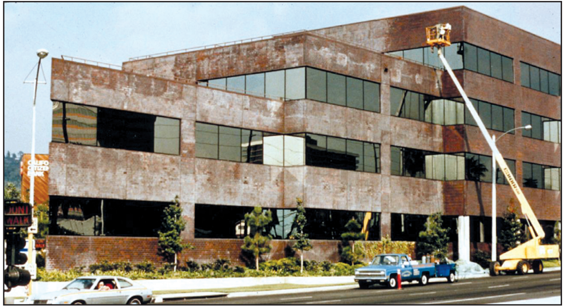
Figure 8: Workers remove sealer blush from a Southern California office building. Sealer blush results from using film-forming sealers on masonry. As water tries to evaporate out of the masonry, it is blocked by the film former. Eventually, the escaping water vapor breaks the sealer bond in spots. Where the sealer has debonded, more water from rain or other sources soaks in, leading to further debonding and more widespread sealer blush. The condition, as shown here, is correctable only by removing the failed coating, which can be expensive. (Photo courtesy of Prosoco.)
