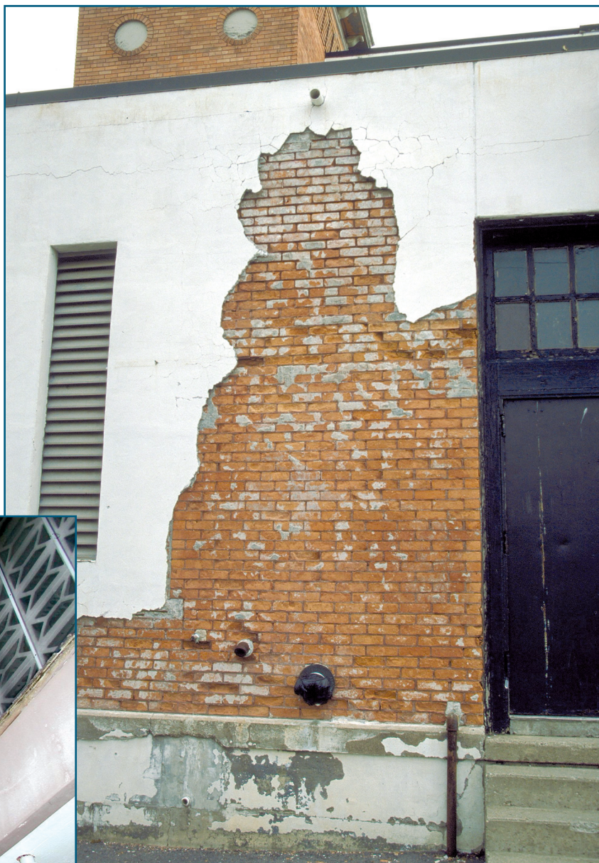
Figure 7: Freeze/thaw brick and parge coating failure.
