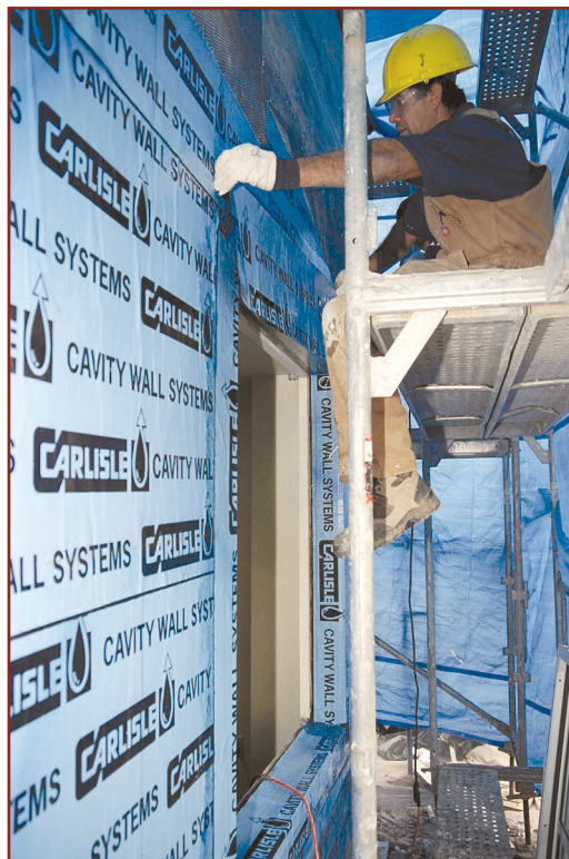
Photo 1: Carlisle Coatings and Waterproofing's 705 Self-adhering Vapor and Barrier System being applied to a new building.
