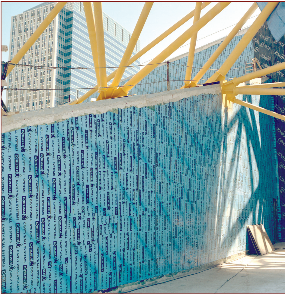
Photo 2: Carlisle Coatings and Waterproofing's 705 Self-adhering Vapor and Barrier System being applied to a new building.
