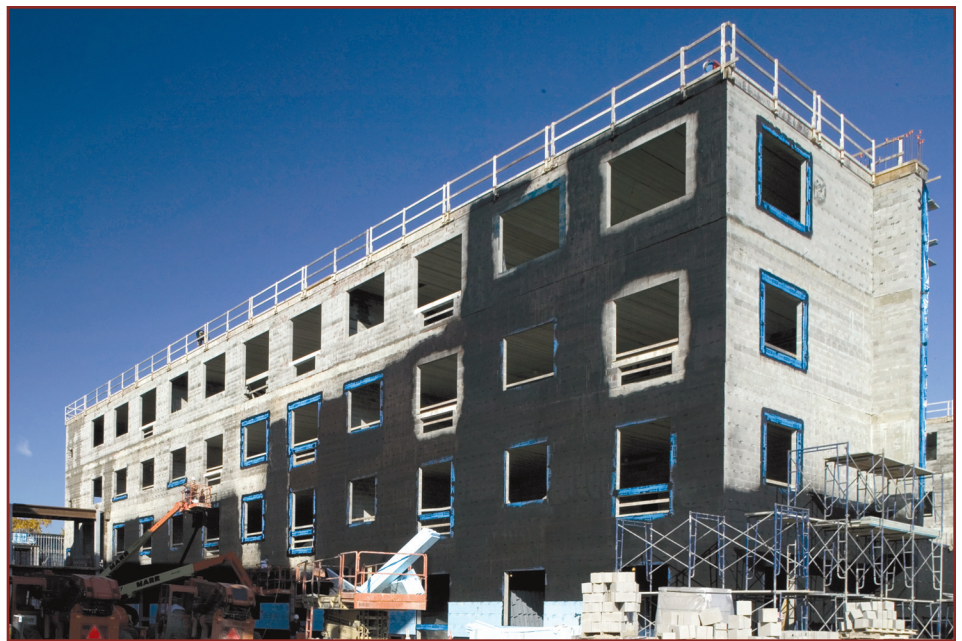
Photo 4: Carlisle Coatings and Waterproofing's Barriseal Liquid-Applied Air Barrier being applied to Lawrence High School in Lawrence, Massachusetts.
