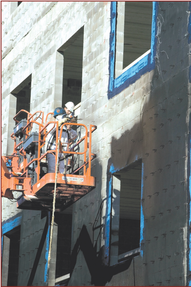
Photo 3: Carlisle Coatings and Waterproofing's Barriseal Liquid-Applied Air Barrier being applied to Lawrence High School in Lawrence, Massachusetts.
