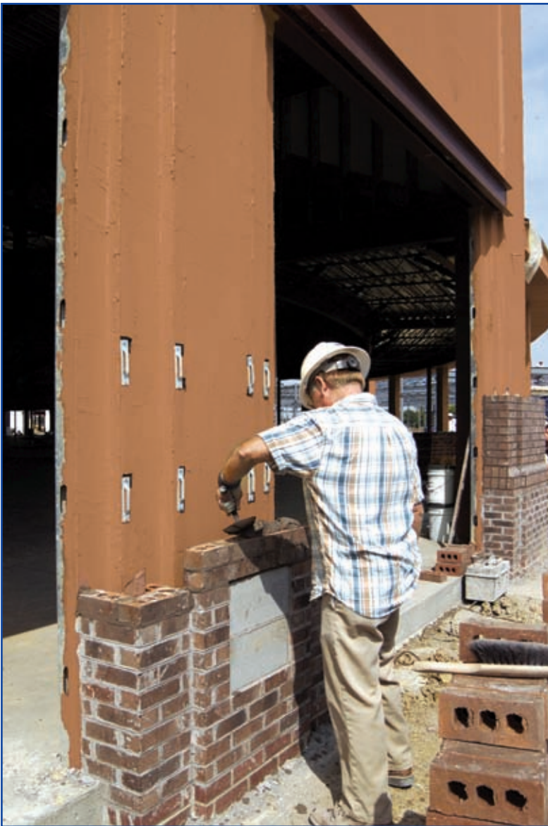
A mason installs a brick veneer over sheathing coated with a water-based, fluid-applied air barrier. (Photo, courtesy PROSOCO.)
