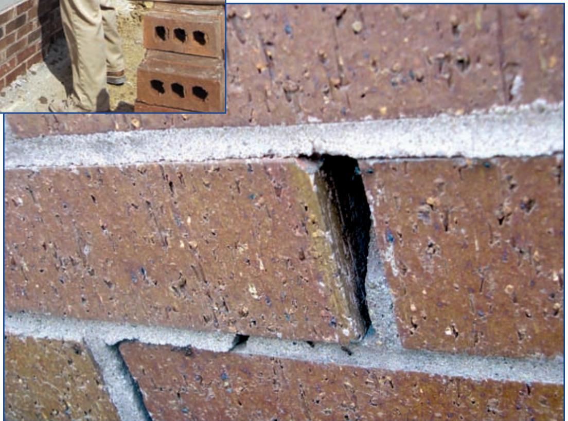
This opening in the masonry veneer lets warm, moist air into the building envelope. If it finds its way through the structural wall, there is danger of condensation in the cooler recesses of the wall assembly. Condensation creates conditions for mold and other wall-component deterioration. Air barriers stop the air flow at the structural walls. (Photo, courtesy PROSOCO.)
