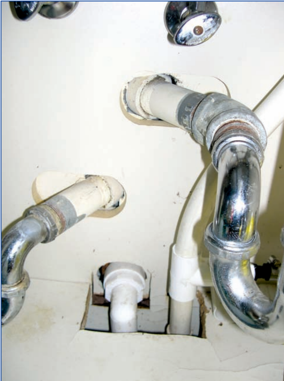
Under a sink, pipes penetrate the wall assembly. Even though the gaps seem tiny, for air, they are a superhighway. If there is a pathway to the outdoors, expensively conditioned air will blow out just the same as if someone opened a door or window. Air barriers block those pathways. (Photo, courtesy PROSOCO.)
