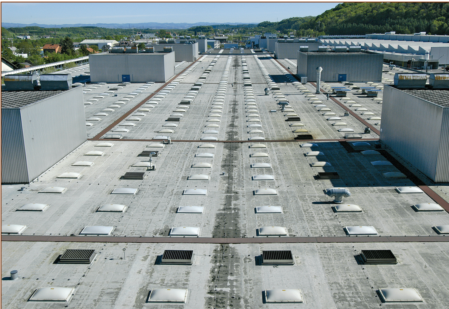
Some 646,000 square feet of liquid waterproofing have been laid over the various roof components on the BMW plant roof in Steyr, Austria, over the last 15 years.
