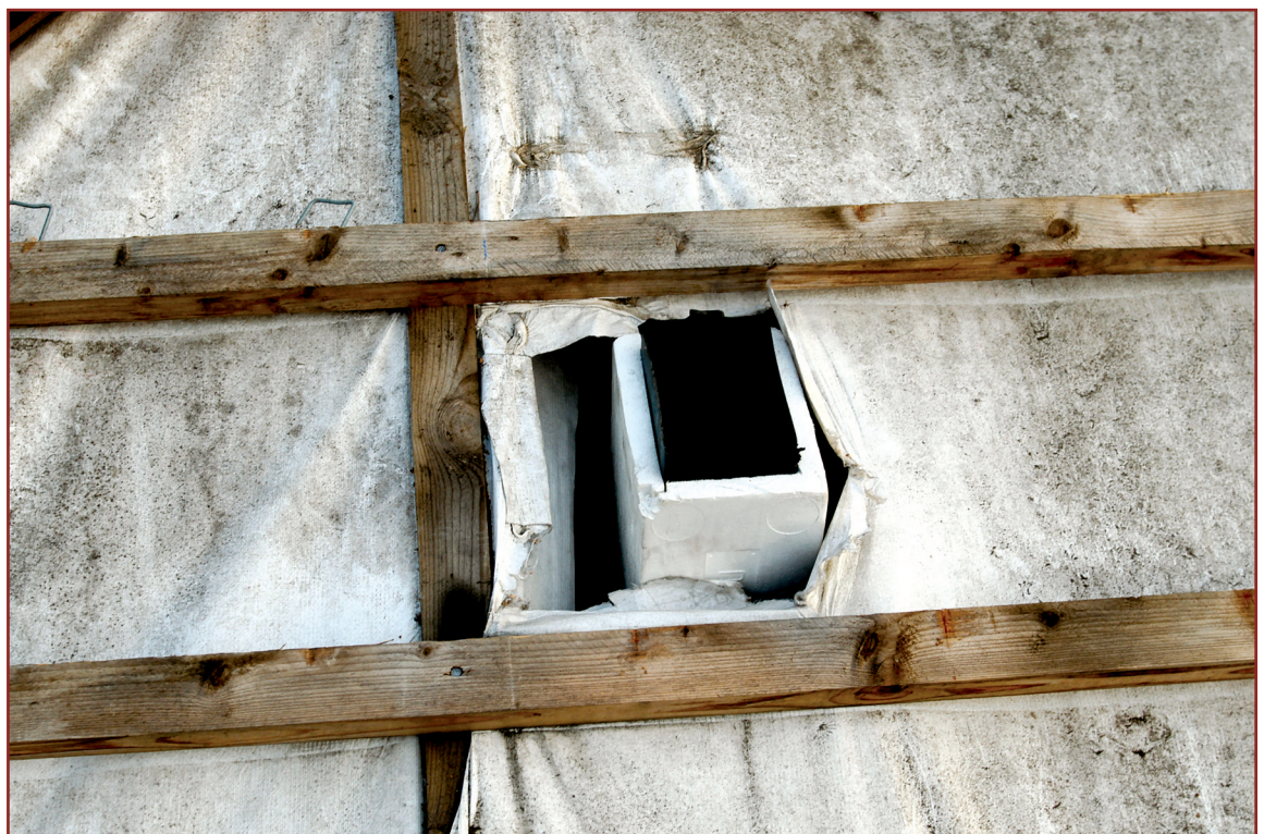
Figure 7 – Example of detail around ventilation duct – very poor workmanship!
