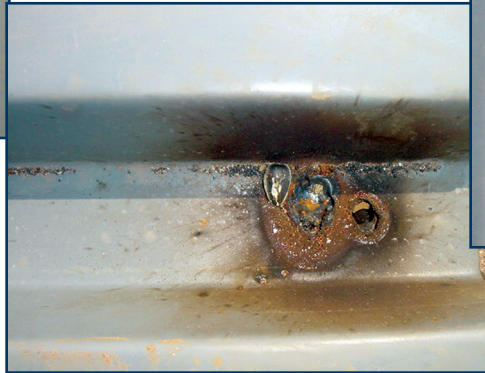
Photo 3 – Really poor-quality weld with blow-through on right side; second attempt was successful, though it is not painted yet.
