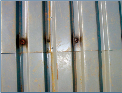
Photo 2 – Missing weld at critical juncture of four pieces of deck that was repaired with screws. The leftmost weld has sheared or failed.
