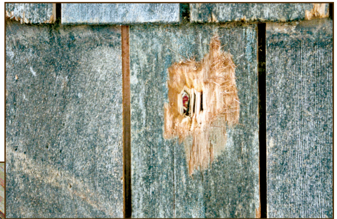
Photo 3C – Actual pressure-washing damage. This type of damage is typically caused by inexperienced equipment users. Contact CSSB for care and maintenance of cedar shingles and shakes.
