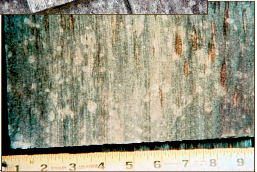
Photo 2C – Many small hail impact marks, but no splits in shingle.
