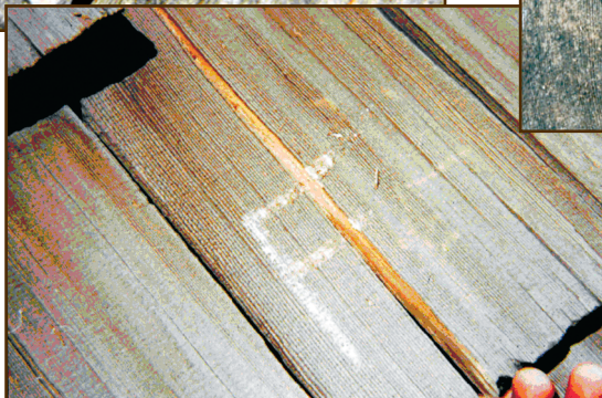
Photo 3B – Footfall split damage (note no denting and new cedar color).
