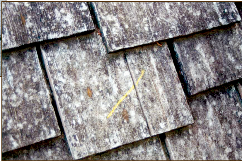
Photo 2B – Weathering split and small hail impact marks.
