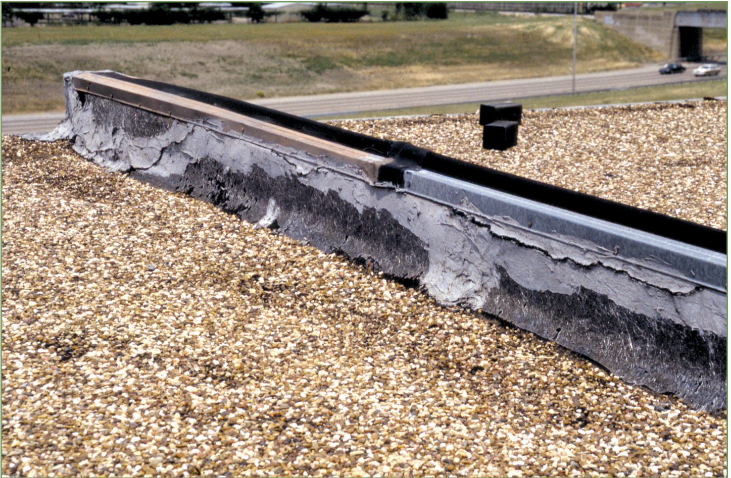
Splits at an expansion joint. Wall movement was not helped by the expansion-joint cover.
