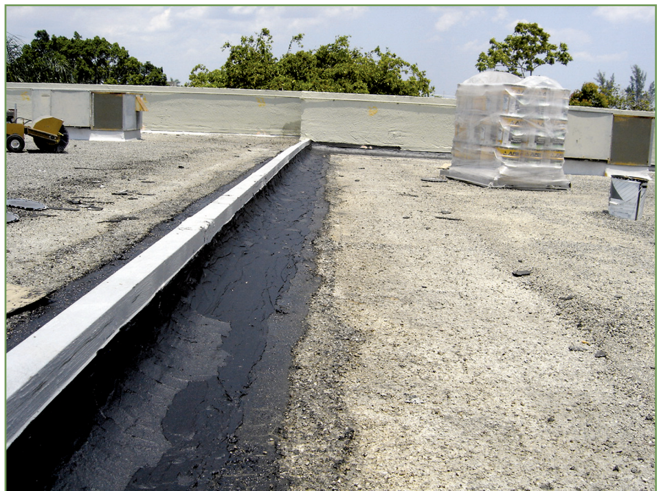
Note the wide spudded area at the base of this roof divider.
