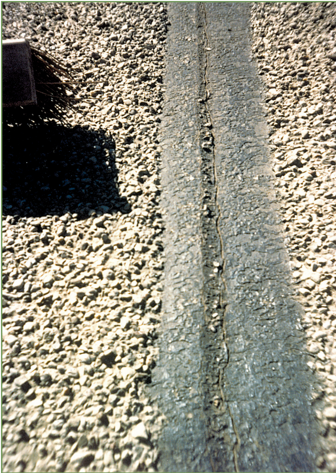
Exposed split at insulation joint.
