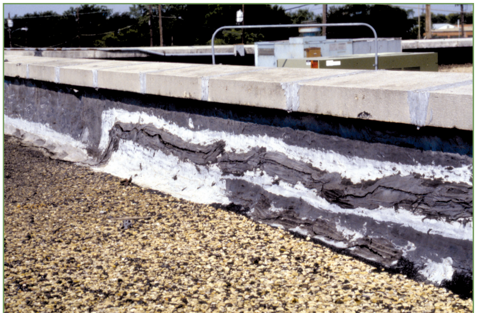
Split in base flashing on concrete block parapet wall.
