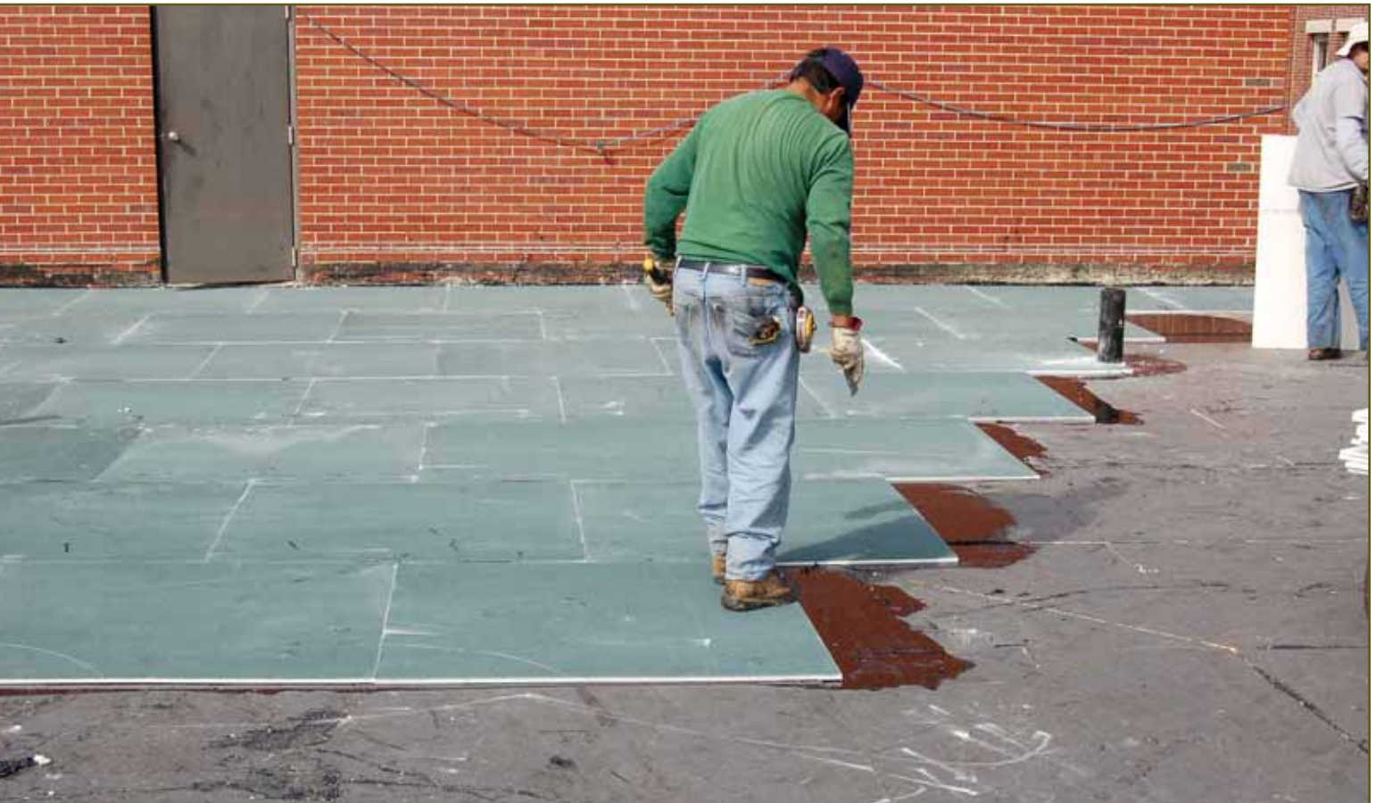
Photo 1 – Long-term design solutions to roofing concerns often involve the work of associated trades. This mechanical penthouse requires complete tuckpointing and masonry restoration work prior to the commencement of roof replacement operations. (Photo by Tom Hutchinson.)
