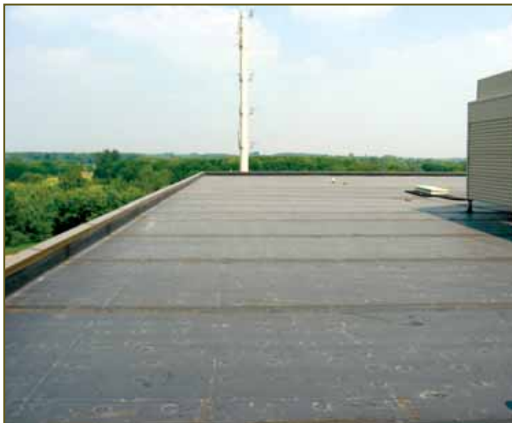
Photo 7 – Another view of the same roof in Photos 5 and 6. Photo by Tom Hutchinson.
