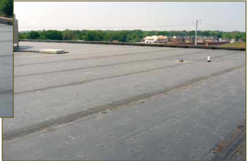
Photo 5 – This three-year-old, 90-mil EPDM roof, designed to FM 1-120 standards, is well on its way to achieving long-term service life (a minimum of 30 years). (Photo by Tom Hutchinson.)
