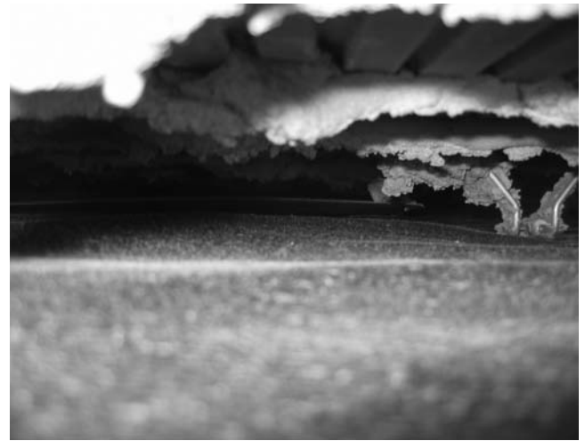
Figure 19 – Mortar bridging at wall tie.
