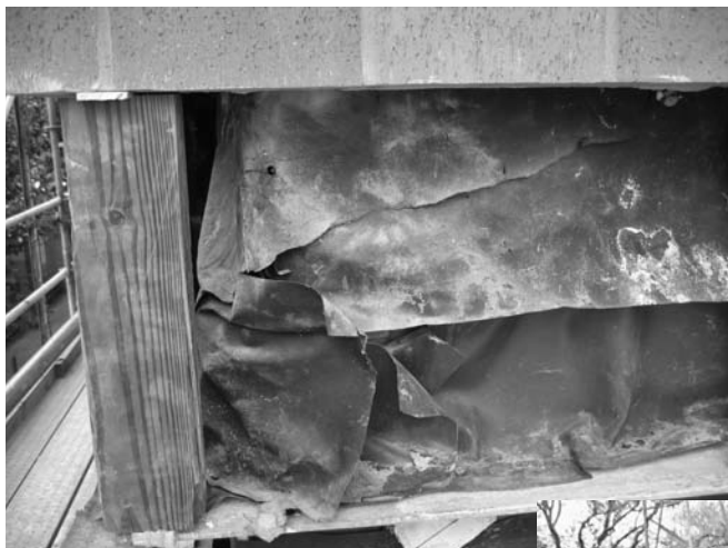
Figure 10 – Improper weather-resistant barrier at corner.
