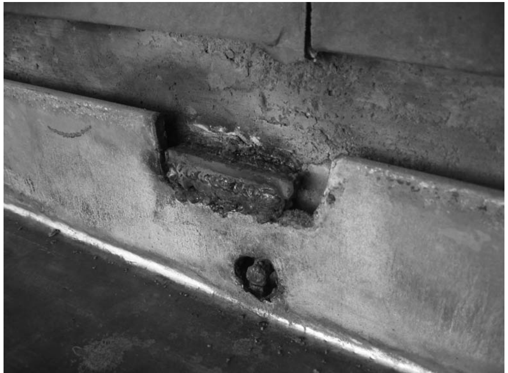
Figure 22 – Improper weld between shelf angle and embed.
