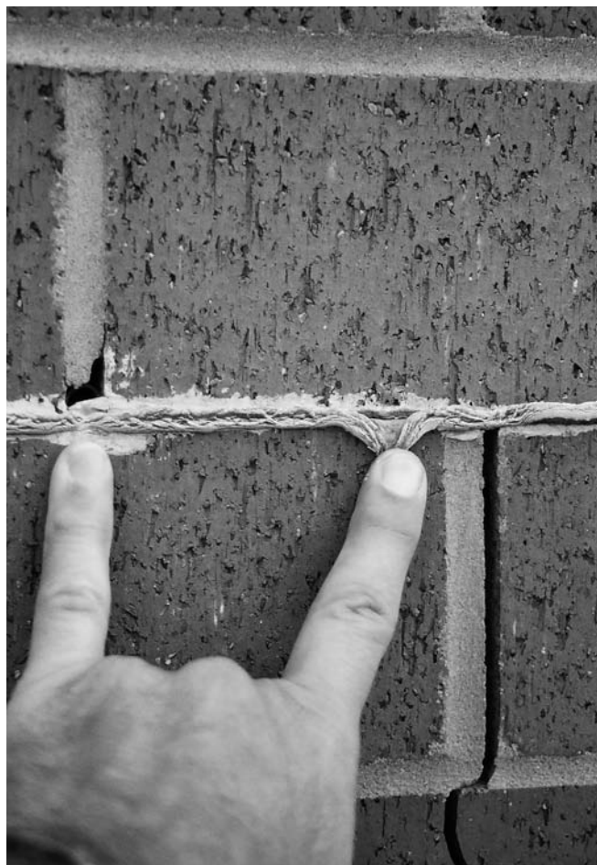
Figure 6 – Sealants failing in compression: masonry cracks.
