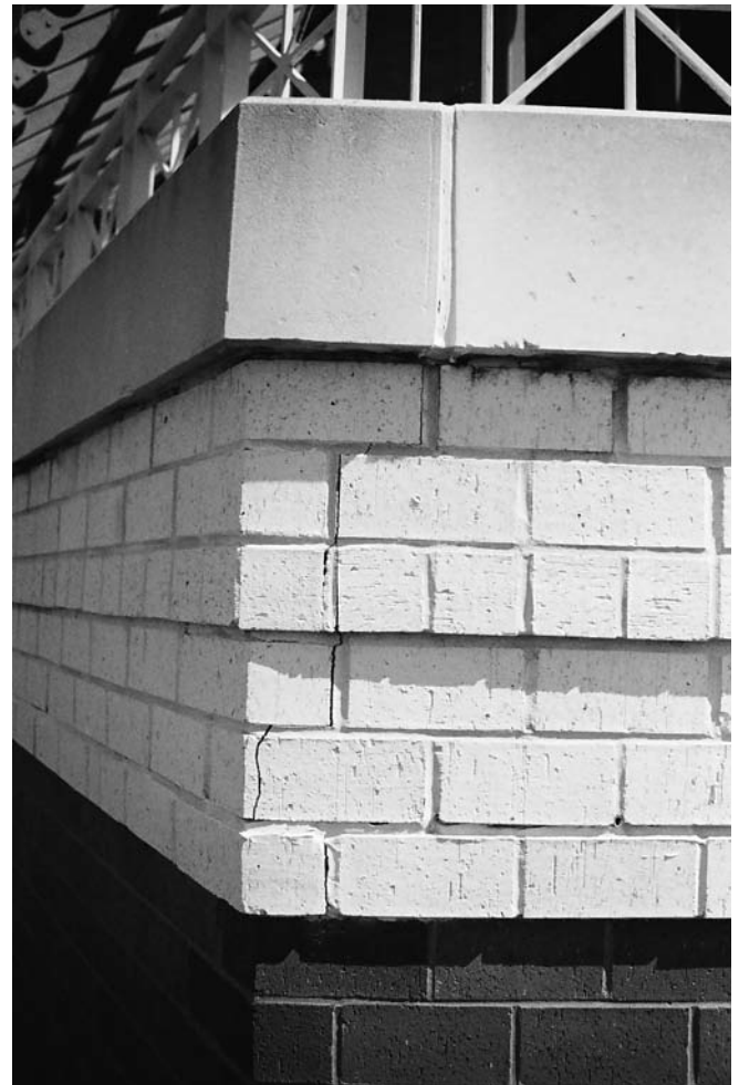
Figure 2 – Cracks in brick veneer at corner.
