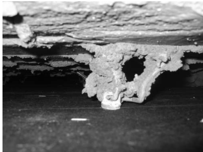
Figure 20 – Mortar bridging at wall tie.
