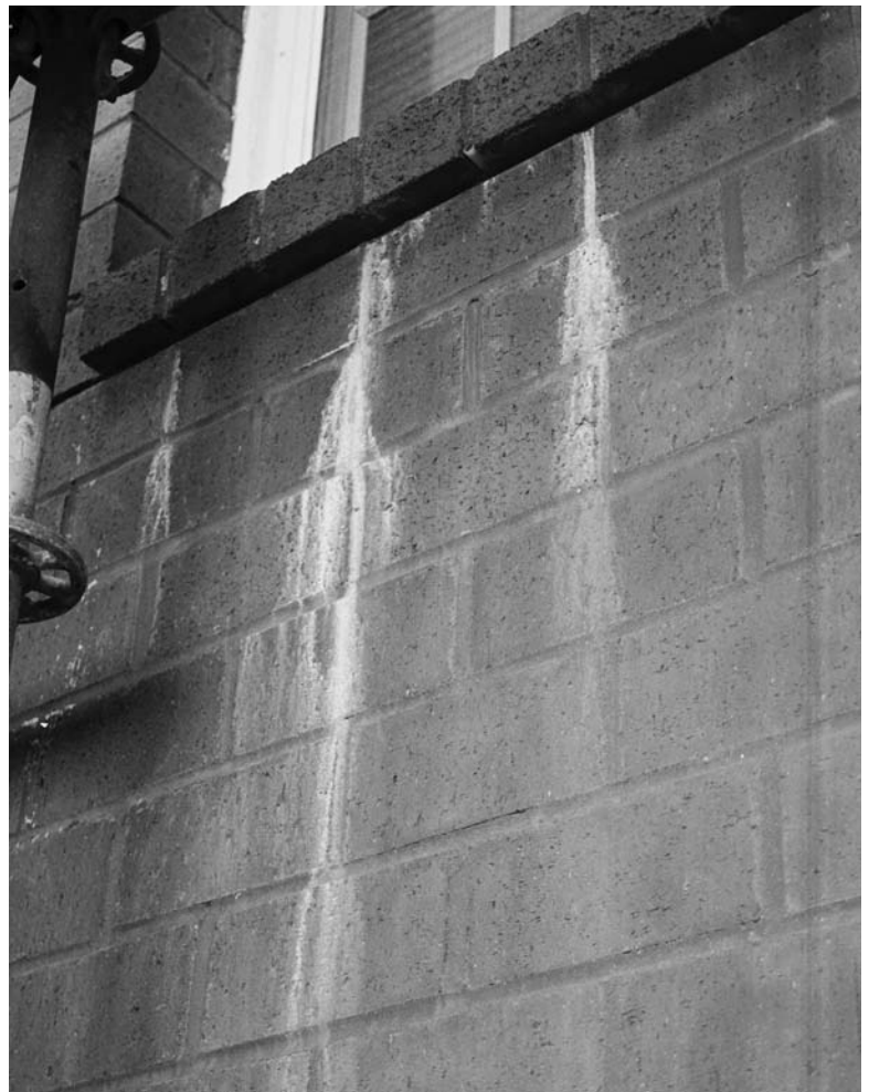
Figure 4 – Efflorescence and water stains below brick sill.
