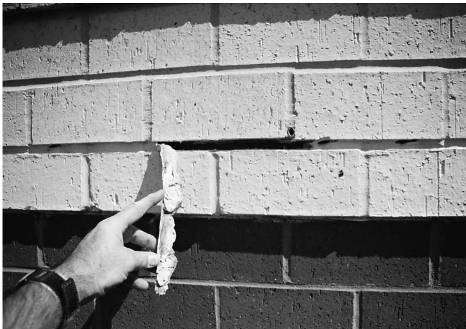
Figure 5 – Sealant installed with no backer rod.
