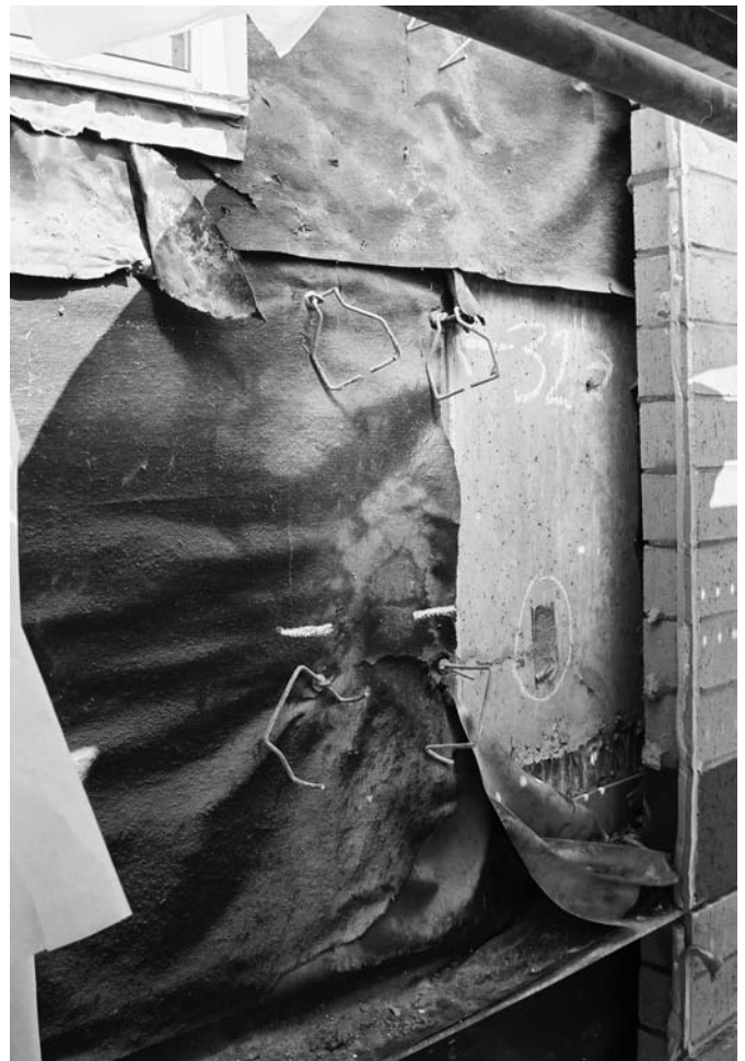
Figure 9 – Weather-resistive barrier stops short of column; not sealed at terminations.
