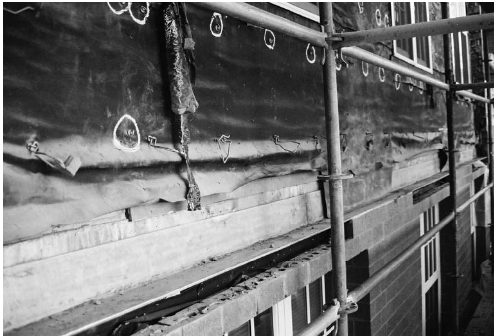
Figure 8 – Weather-resistive barrier not integrated with shelf angle; missing wall ties.
