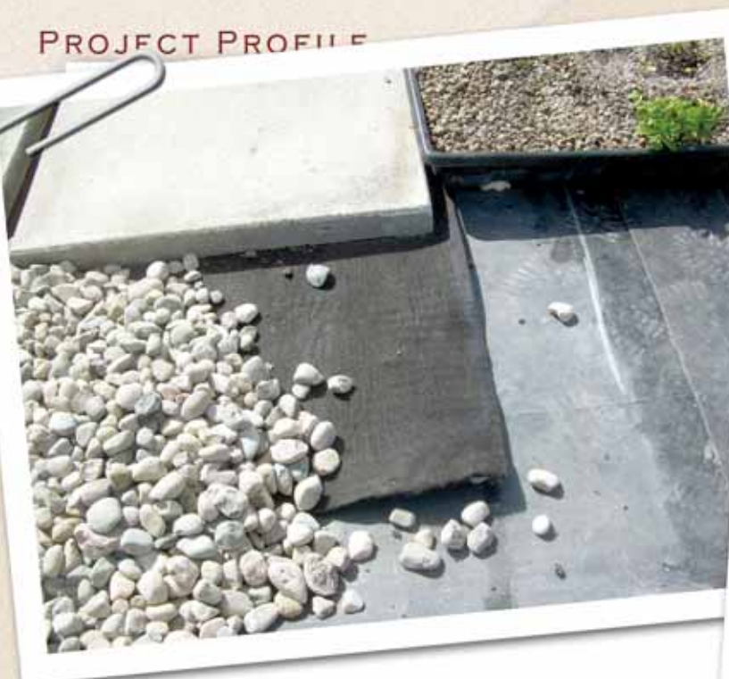
Shown are the construction material layers: waterproofing membrane, drainage and water retention mat, and green roof tray. Pavers and ballast are used in the nongreen areas.
