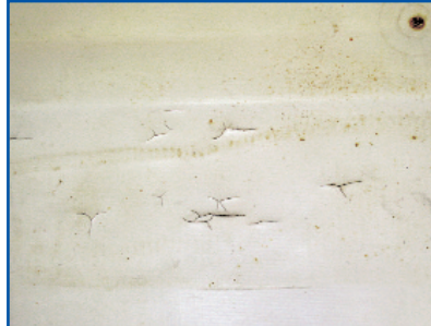
Photo 33 – View of damage on bottom of membrane.
