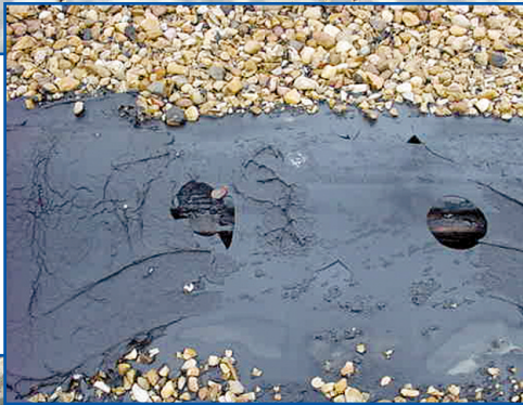
Photo 9 – Punctures in weathered expansion joint.
