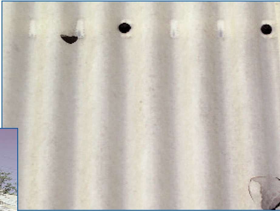
Photo 20 – Puncture in corrugated fiberglass panel.
