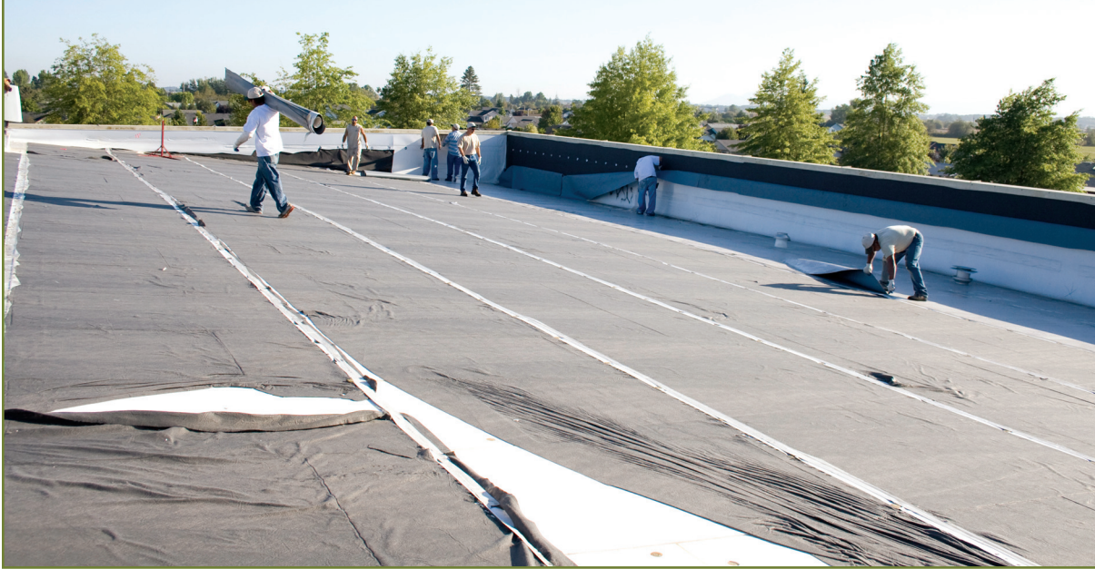
Contractors segregate the fasteners from the seam strips after the main vinyl sheets have been removed from the substrate. Image courtesy Vinyl Roofing Division, CFFA.
