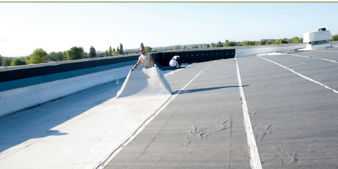
Contractors easily lift a flexible sheet of retired membrane from the roof to be rolled in preparation for transport off site. Image courtesy Vinyl Roofing Division, CFFA.
