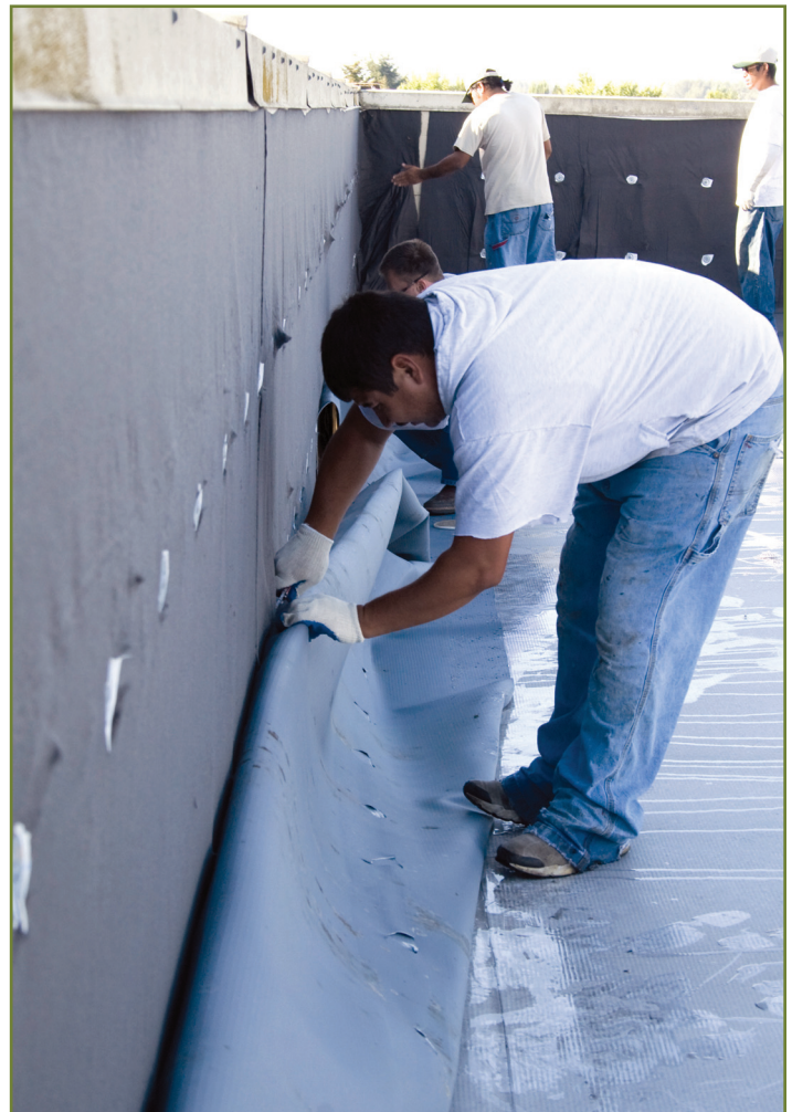
Contractors separate the vinyl membrane from the wall fasteners and plates, which will also be recycled. Image courtesy Vinyl Roofing Division, CFFA.
