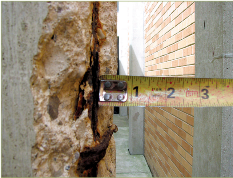
Figure 3 – Lack of concrete cover.
