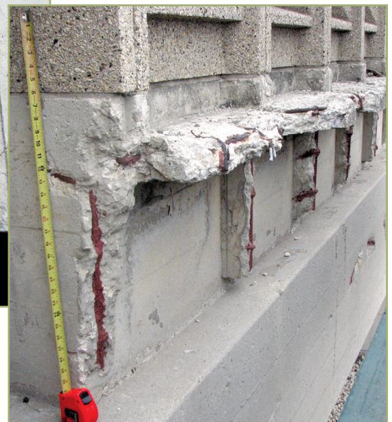
Figure 5 – Spalls in concrete.
