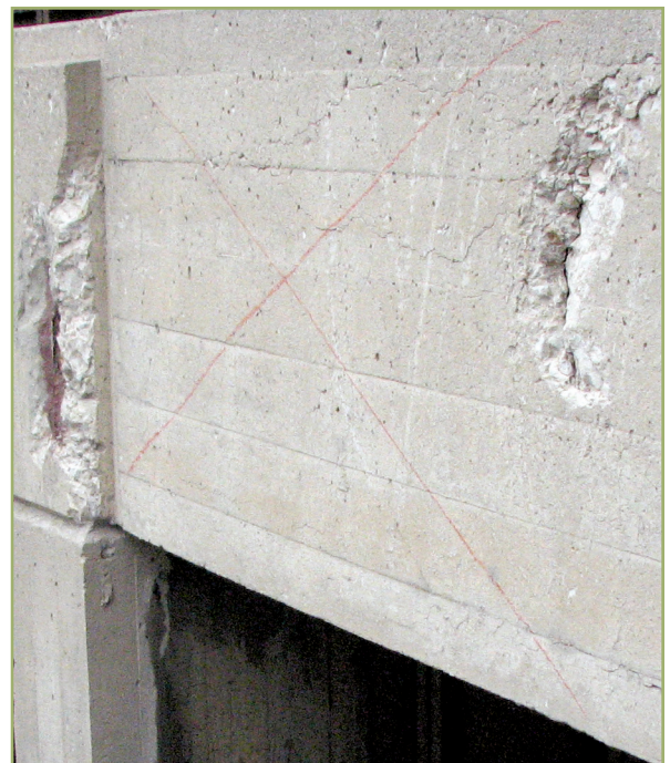
Figure 9 - Area of distress discovered by sounding.
