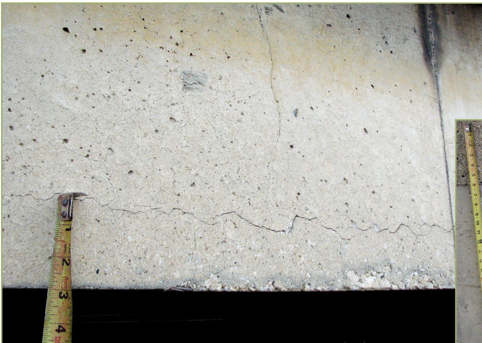
Figure 4 – Cracks in concrete.
