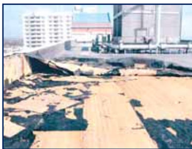
Hurricane Charley. Severe wind damage with weak bond between membrane and insulation. Photo, courtesy of Tecta America.
