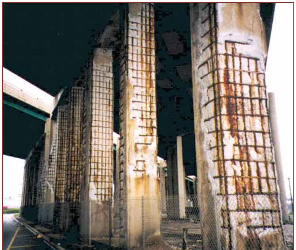
Photo 2 – Spalling of concrete due to chloride attack of embedded reinforcing steel
