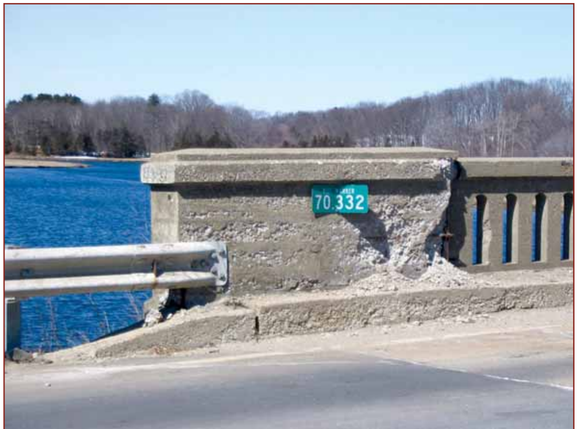
Photo 4 – Freeze/thaw damage to a bridge wing wall
