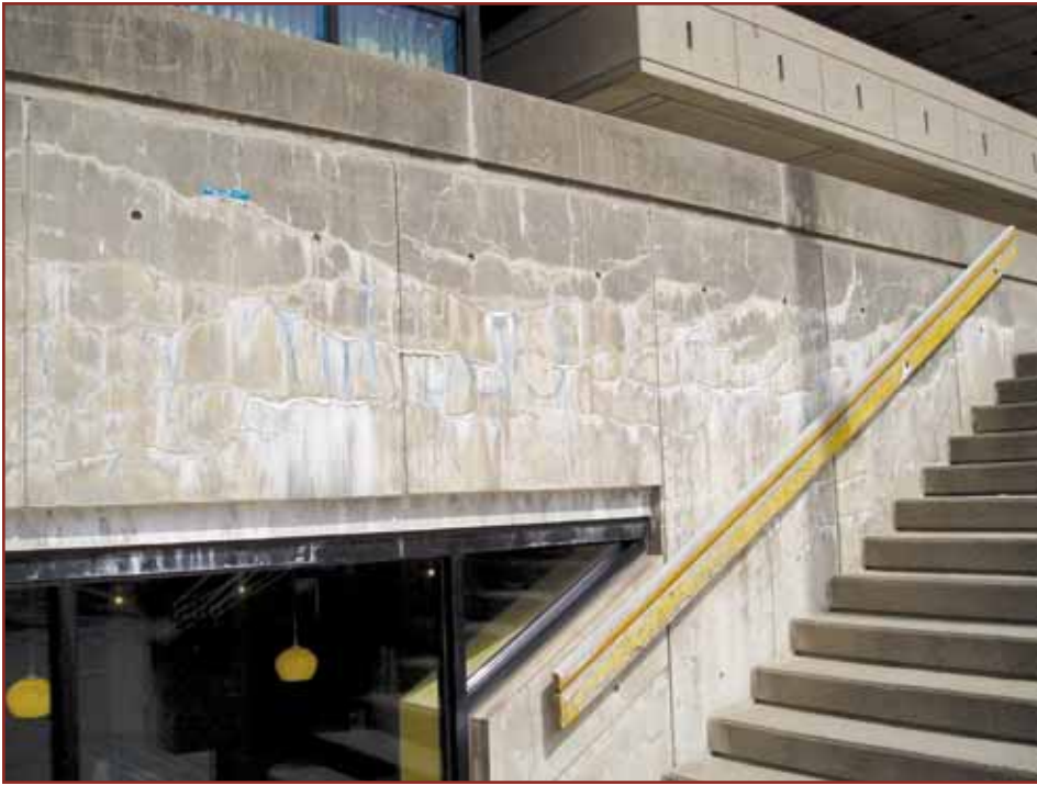
Photo 3 – Alkali-silica deterioration of parapet wall
