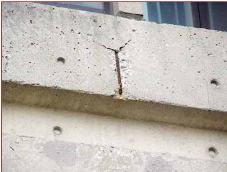
Photo 1A – Corrosion of embedded steel
