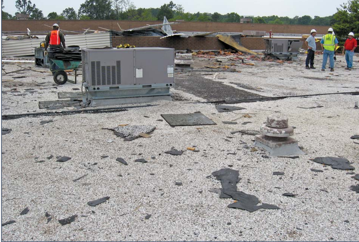
Figure 2 – The roof area on the other side of the short parapet wall from the truck bay. All debris is from the truck bay roof. The roof and gravel on this area stayed intact.
