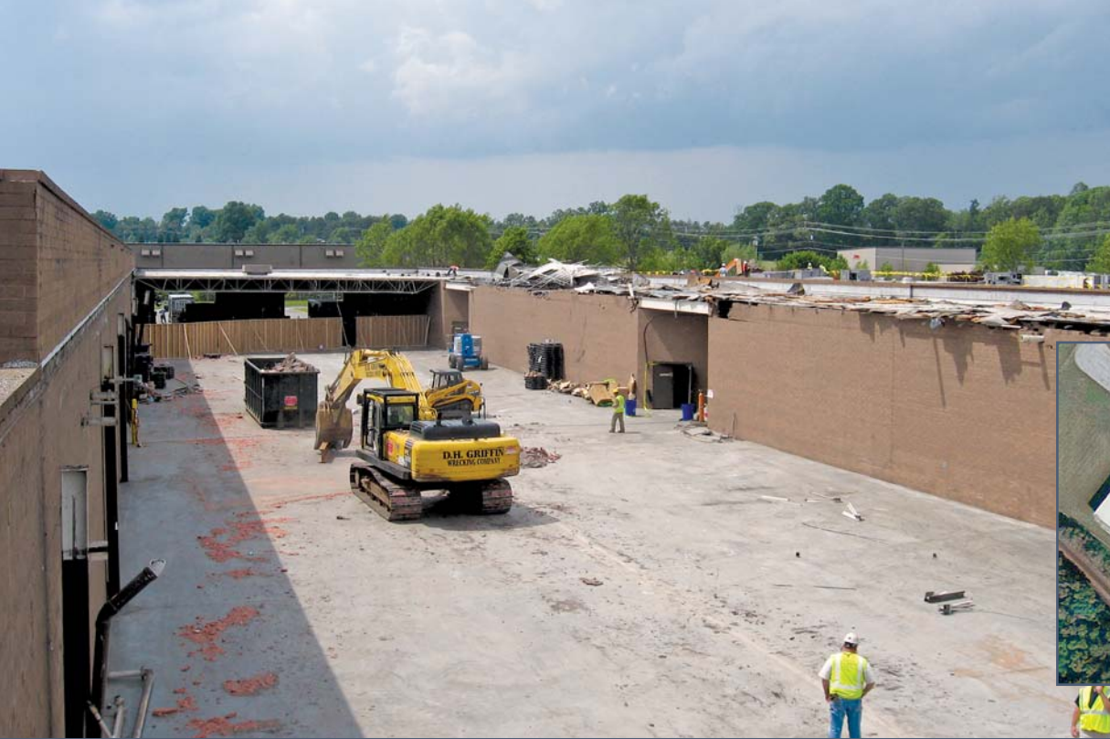
Figure 3 – The entire roof structure over the truck bay, except for the last few feet, was destroyed. Just a few feet from where the structure was ripped away, the 26-year-old BUR remained intact.
