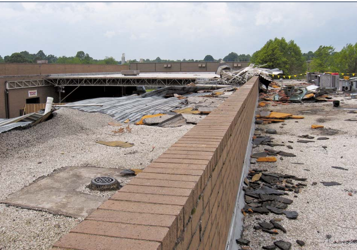
Figure 1 – The warehouse area to the side of the truck bay. Note that the BUR stays intact on the deck even as the deck is bent up by the force of the wind.
